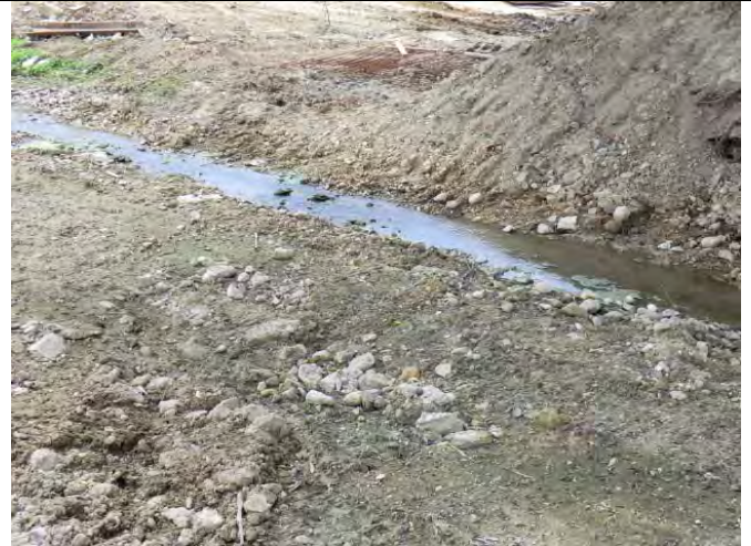
Debris in channel has been removed and the riversides have been compacted against soil erosion. (MUP05)
