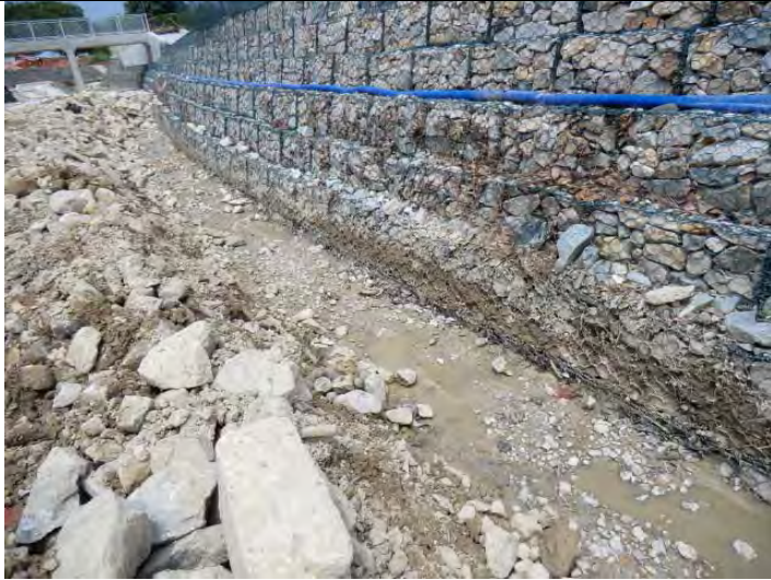
Photo 1: Drainage channel has been diverted in order to prevent occurrence of muddy water [TKL07]
