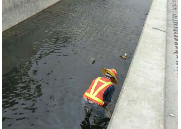
Photo 2: Refuse was being removed from the channel.. [TKL07]
