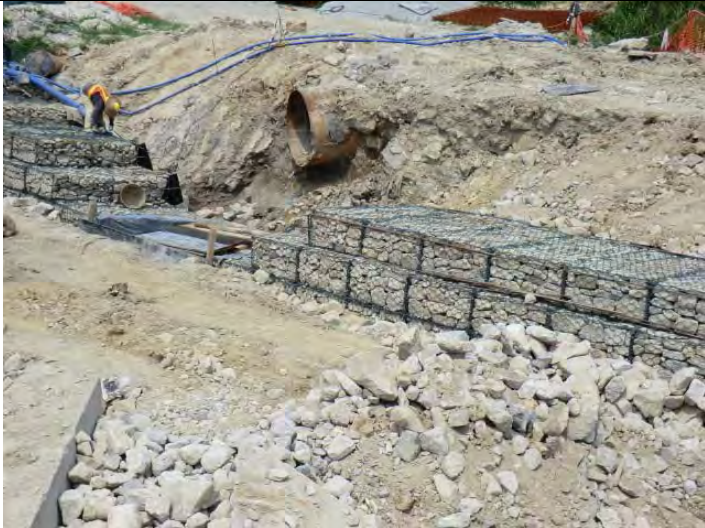
Photo 1: A ponding of muddy water was eliminated. By water diversion using pipeline.
