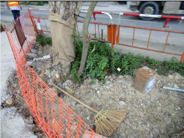
Photo 1: Free standing chemical container without drip tray was observed, the contractor was reminded to provide drip tray for all chemical containers on site.
