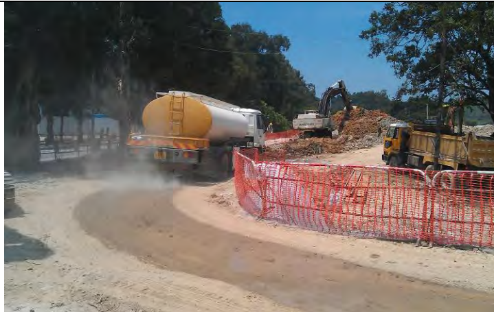
Photo1: Spraying water on dry haul road was observed.
