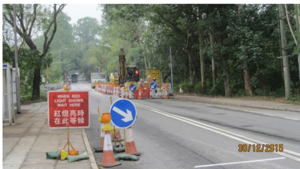
Excavation work using excavator at nearby works site with temporary traffic arrangements on Sha Tau Kok Road
