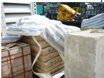
Photo 1: Cement bags near entrance of noise enclosure were covered improperly
