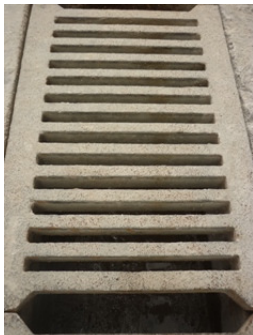
Photo 6: The U-channel had been cleared
