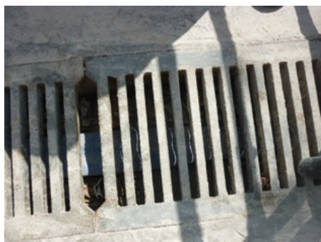
Photo 1: The U- channel near noise enclosure was found with accumulated leaves and mud
