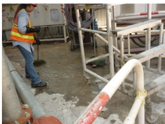
Photo 5: Worker was clearing the accumulated water near the site hoarding during site inspection.
