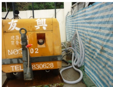
Photo 2: Oil spot was found near the generator
