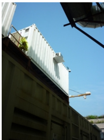
Photos 1: No improvement on the leaking air-conditioner since last inspection
