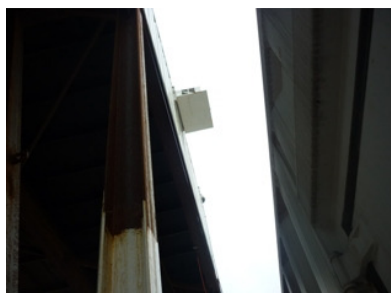
Photo 1: The water leakage was found from air conditioner.
