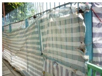
Photo 1: Broken sailcloth was found along the site boundary
