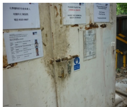
Photo 2: An unlocked chemical waste storage was found
