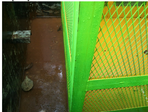
Photo 1: Accumulated water was found in the drip tray
