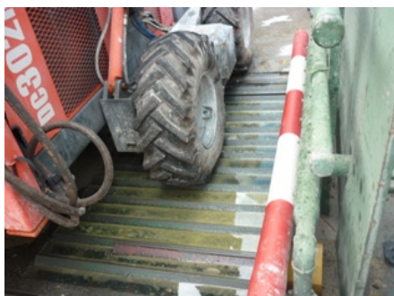
Photo 1: Water accumulation was found in wheel washing facilities
