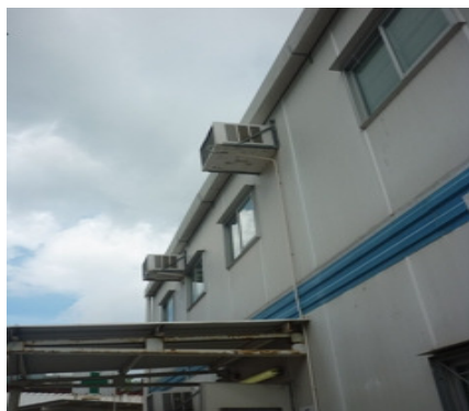
Photo 3: Waste water leakage was found from air-conditioner.
