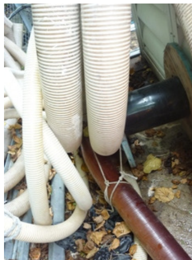
Photo 2: Leaves and water accumulation was found behind the generator
