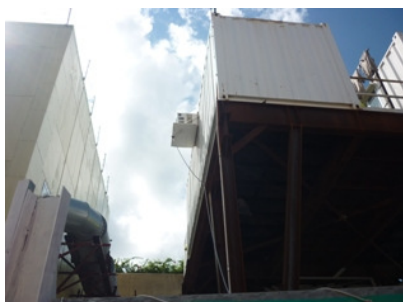
Photo 1 Water leaking from air conditioner and waste water accumulated near the EP notice board
