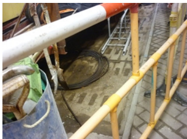
Photo 1 The accumulated water near the entrance of noise enclosure was cleared
