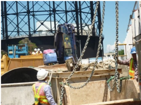
Photo 1: The smoke emission from excavator was found near the exit
