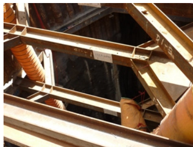
Photo 2 The accumulated water which found on the I-bar in the site was cleared
