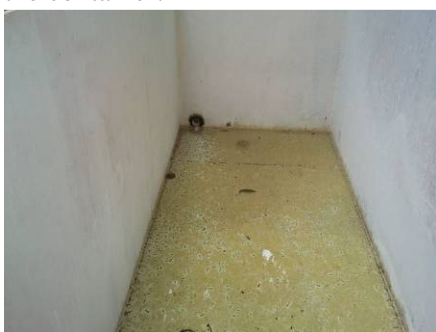
Photo 1 The accumulated water was found in the container.
