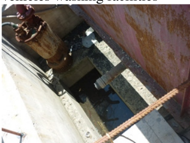
Photo 3: The rubbishes were found in the pit near vehicles washing facilities
