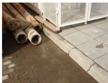
Photo 2: Water accumulated in works area near
