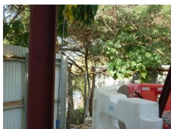
Photo 1: Part of site boundary without metal hoarding was found
