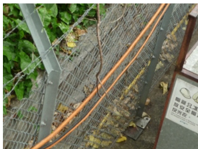
Photo 1 Accumulated leaves were found in U-channel that behind the fence boundary
