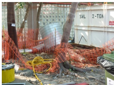
Photo 1: Damage tree protecting fence was found
