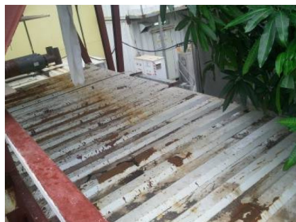
Photo 2 The accumulated water was found on the top of container.
