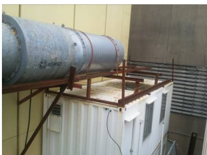
Photo 3 Unused chemical materials were removed on roof of workers rest area.
