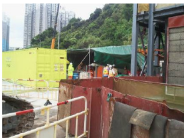
Photo 1 The 3-sides cover at the cement mixing area was found improperly.
