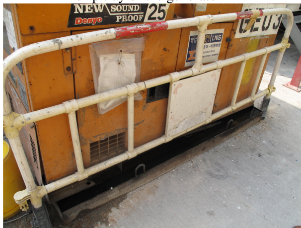
Photo 2 Water accumulation was found in the drip tray of the generator
