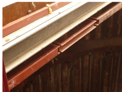
Photo 2 Some acoustic material missing was observed between the noise cover
