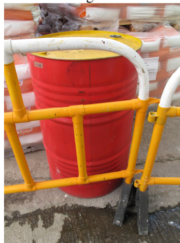
Photo 2 Chemical drum without drip tray found in worker resting area near the entrance
