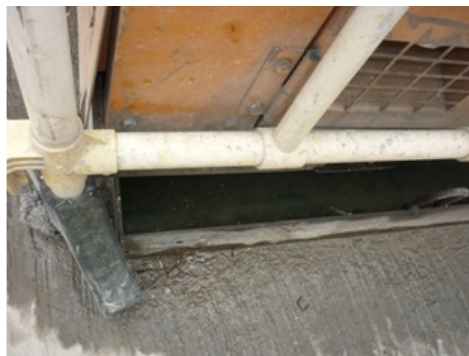
Photo 2 Water accumulation was found in the drip tray of the generator near the noise enclosure
