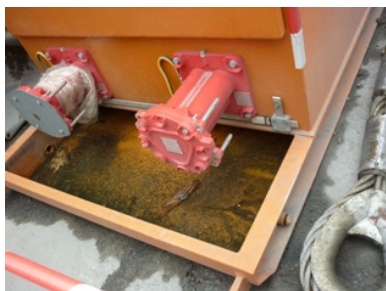
Photo 1 and 2 Water accumulation was found in generator 's drip tray and next to noise enclosure
