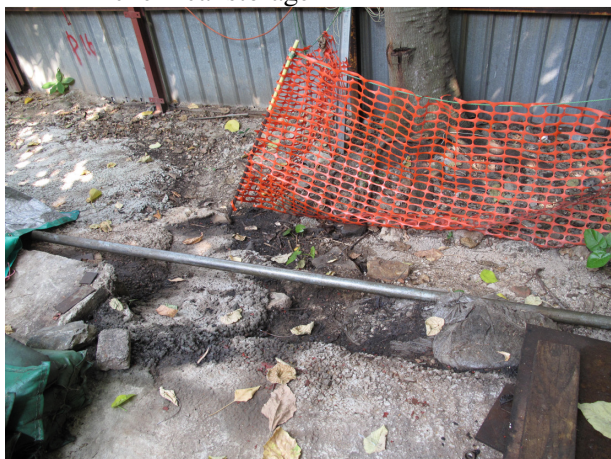
Photo 1 Oil spots were found in the soil near the chemical storage
