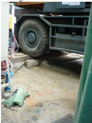
Photo 1 The contractor is recommended to provide drainage for site runoff
