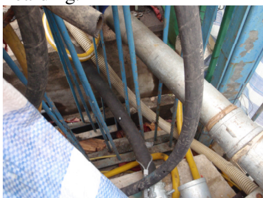
Photo 1 Some general refuses were found in the U-channel near the site hoarding.
