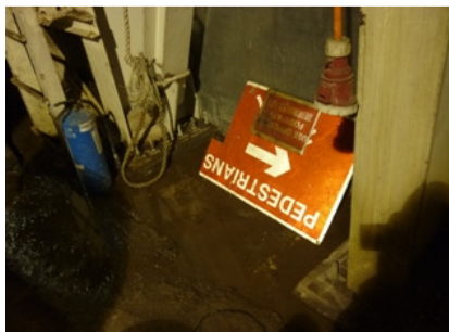
Photo 3 The accumulated water was found on the floor under the air compressor inside the noise enclosure.
