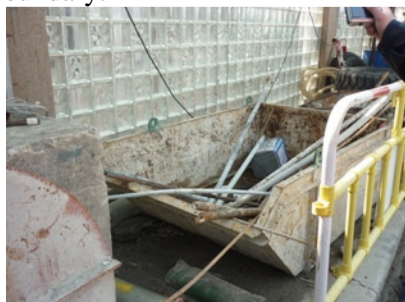
Photos 3 Accumulated water was found in skip near the boundary.
