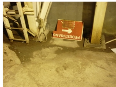
Photo 4 The accumulated water was cleared on the floor under the air compressor inside the noise enclosure.
