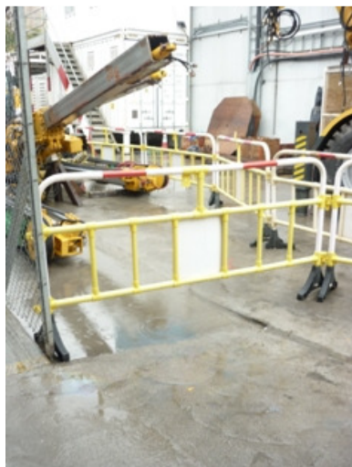
Photos 3 and 4 Oil stain was found near the plant
