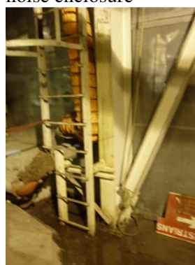
Photo 4 Accumulated water was found on the floor under the air compressor inside the noise enclosure
