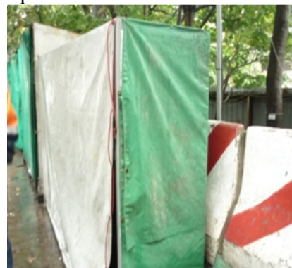
Photo 2 A chemical storage container was found without drip tray and properly labels since last inspection
