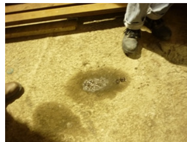
Photo 2 Oil stains were found on the floor at the corner inside the noise enclosure.
