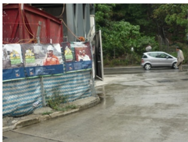
Photo 5 The muddy water near the boundary behind the sedimentation tank was cleared
