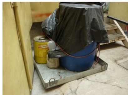
Photo 4 The accumulated water was cleared in the drip tray near the noise enclosure.
