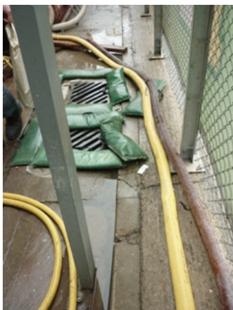
Photo 1 Oil water was found flowing into gully near Aqua. Sed tank
