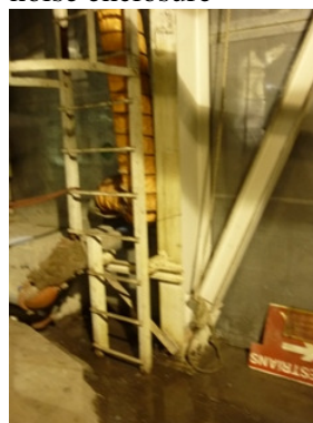
Photo 4 Accumulated water was found on the floor under the air compressor inside the noise enclosure
