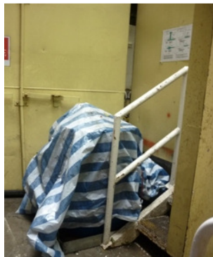
Photo 5 Water accumulation was found in drip tray near the entrance of noise enclosure
