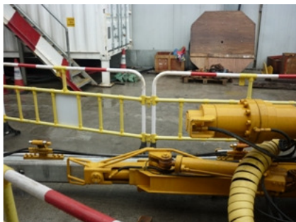
Photo 5 Oil stain on the floor in front of site office was cleared
