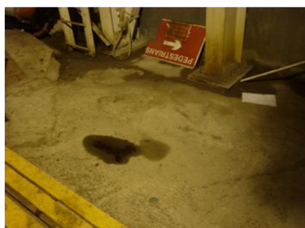
Photo 3 Oil stain was found in the noise enclosure under the air compressor.
