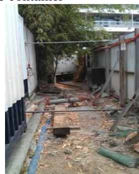
Photo 2 Leaves accumulation was found in the pit behind the container
