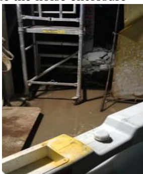
Photo 1 Water accumulation was found near access inside the noise enclosure
