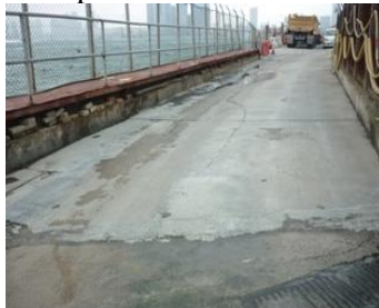
Photo 1 Some stagnant water was found near the access path
