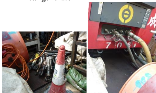
Photo 2 Stagnant water was found in drip tray near generator
