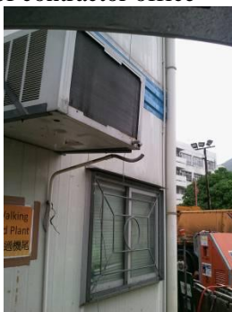
Photos 3 The damage pipe was found of air conditioner of contractor office
