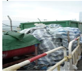
Photo 2 Some cement bags were found without proper cover.
