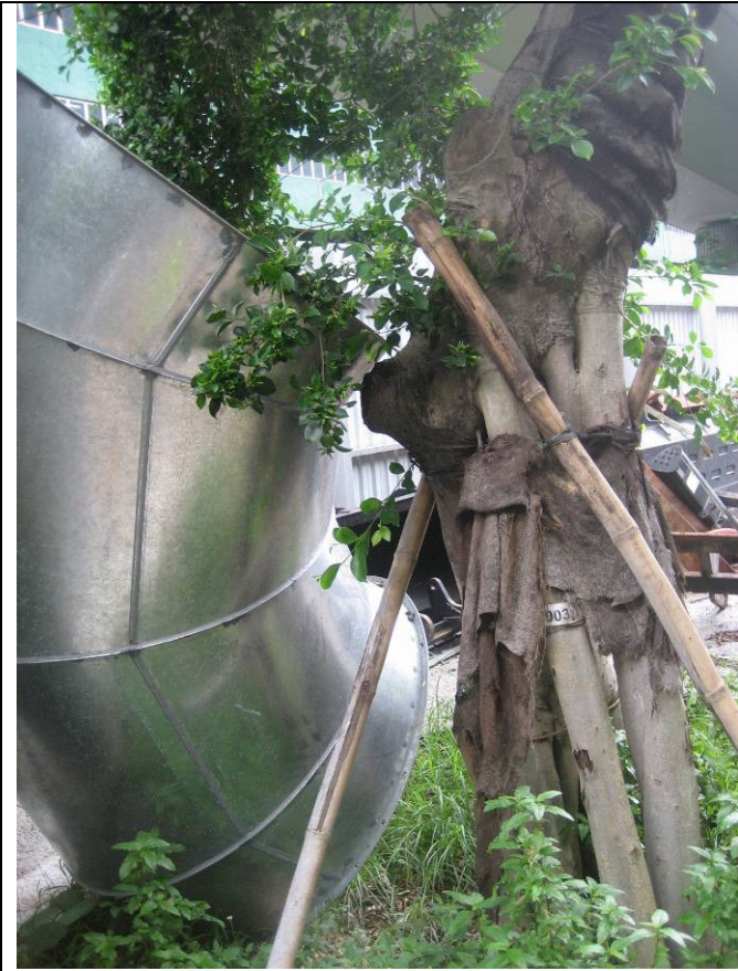
Aberdeen site --- Photo 11 Construction material was observed stored very close to the retained tree T003(T).
