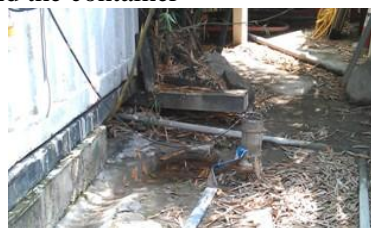
Photo 2 Leaves accumulation was found in the pit behind the container
