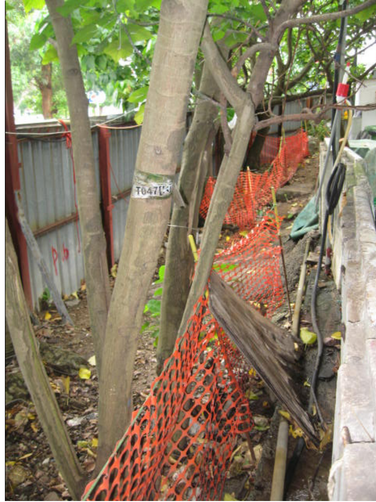
Sandy Bay site --- Photo 6 Construction materials were found stored close to the roots of retained Tree T047 (R).
