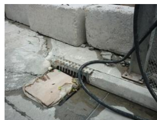
Photo 2 No more contaminated water leaking into the gulley
