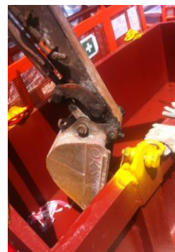
Photo 2 The contractor is reminded to remove stagnant water and rubbish inside the skip.
