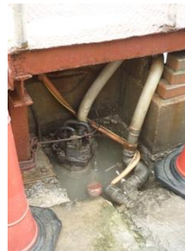
Photo 4 Dilapidation pile was found near the access
