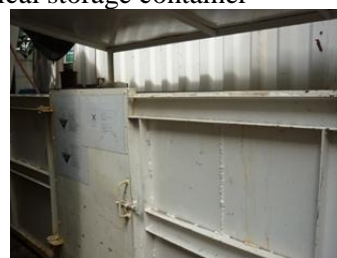
Photo 2 Water accumulation was found in chemical storage container
