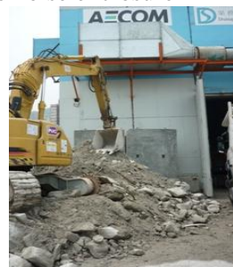
Photo 2 Sand pit without cover or pre-wetting near the noise enclosure
