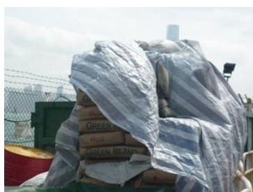
Photo 1 Some cement bags were found without proper cover
