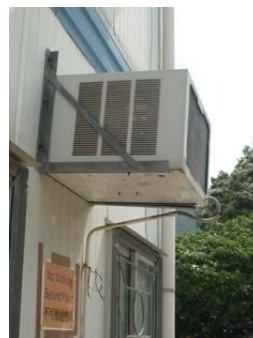
Photo 6 The contractor was reminded to repair the pipe of air conditioner in PTW
