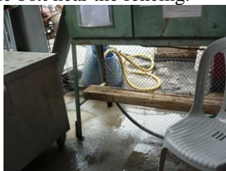
Photo 1 Water accumulation was found near the electric box near the fencing.
