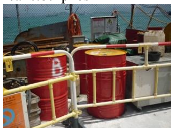
Photo 1 Chemical barrels without drip tray were found near stockpiles
