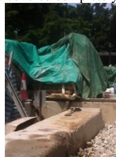
Photo 2 Covers for cement packs were found not to be covered completely
