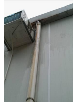
Photo 2 The water leakage was found at the roof of site office
