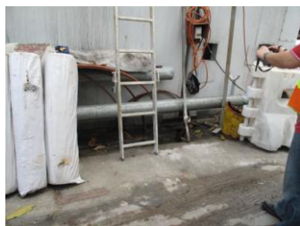
Photo 5 Stagnant water found on tarpaulin near chemical storage area
