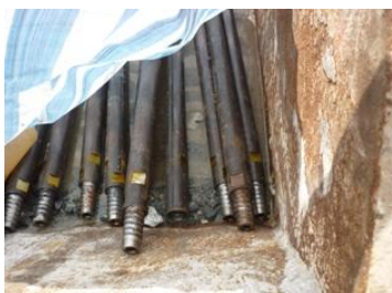
Photo 1 Water accumulation was found in skip on the noise platform
