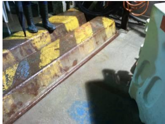
Photo 1 Water accumulation was found near access inside the noise enclosure
