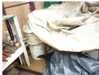
Photo 2 Stagnant water was found in drip tray near generator
