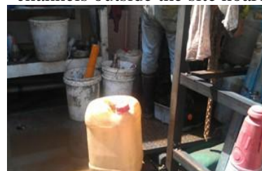
Photo 2 Some trashes were found in the U-channels outside the site hoarding
