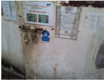
Photo 5 Water accumulation on the top of the empty oil barrels in the fuel storage area
