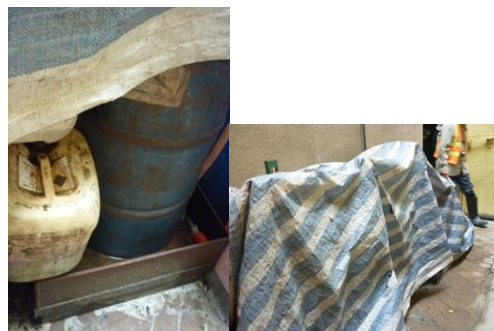
Photo 2 Stagnant water was found in the trip tray near the noise enclosure
