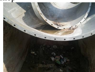
Photo 2 The accumulated water was found on the unused materials in the site area of workshop
