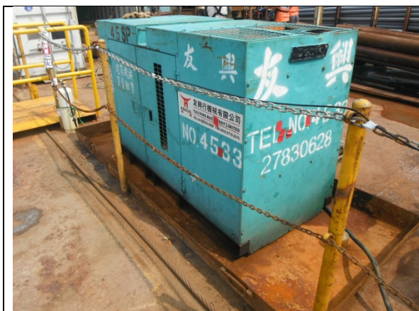
Generator on vessel board
