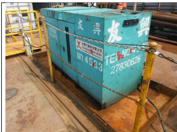
Generator on vessel board
