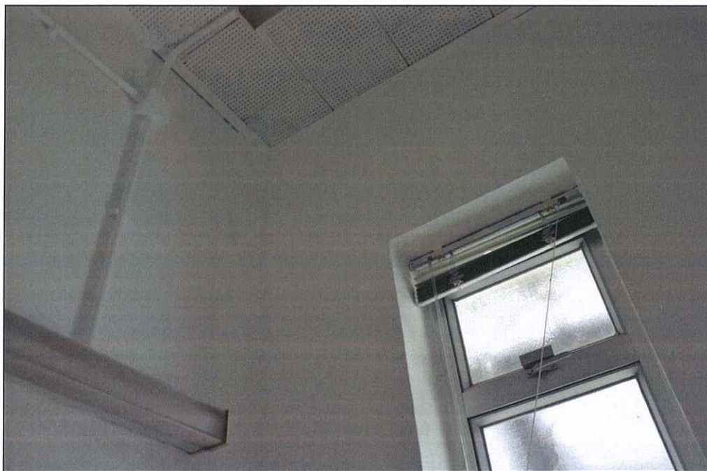
Photo 18.33 – Toilet (wash basin only) at Room 1, ceiling (2011/08/13)
