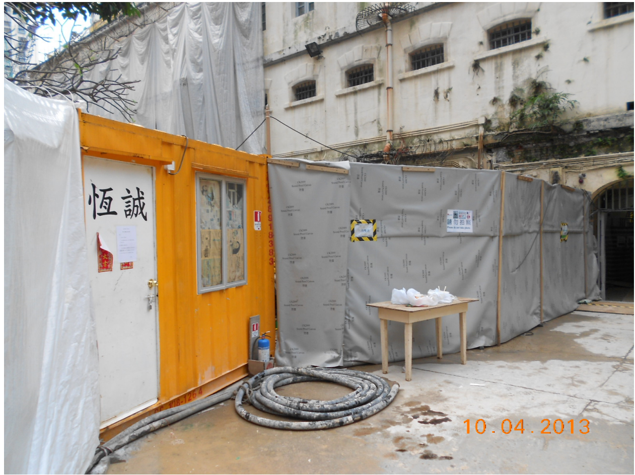
Figure 2 – Noise barrier for air compressors near Block 14
