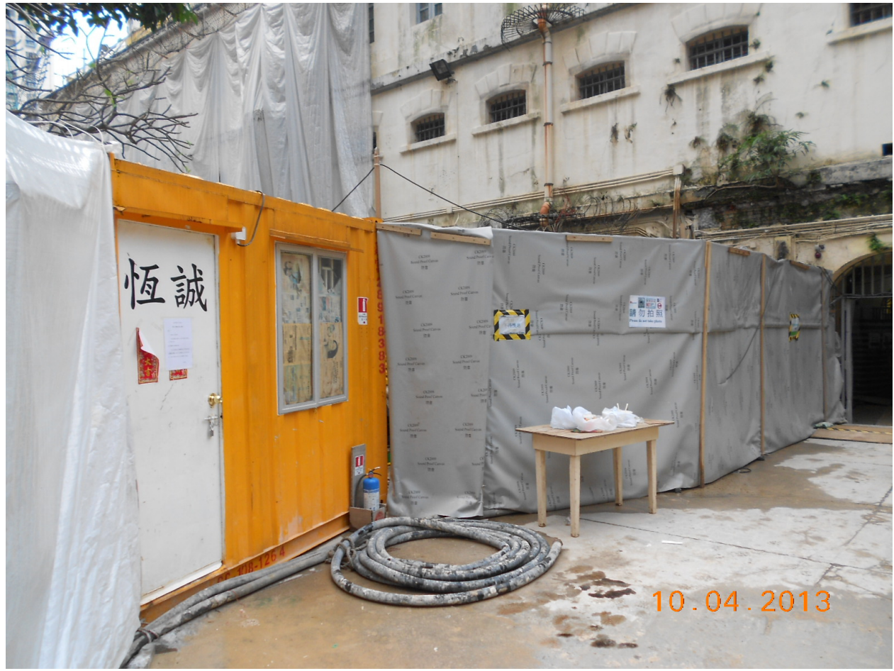
Figure 2 – Noise barrier for air compressors near Block 14
