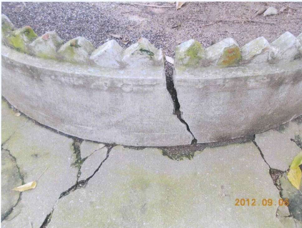
Fig. 3 Cracks are getting worse, remedial work for these cracks are recommended.
