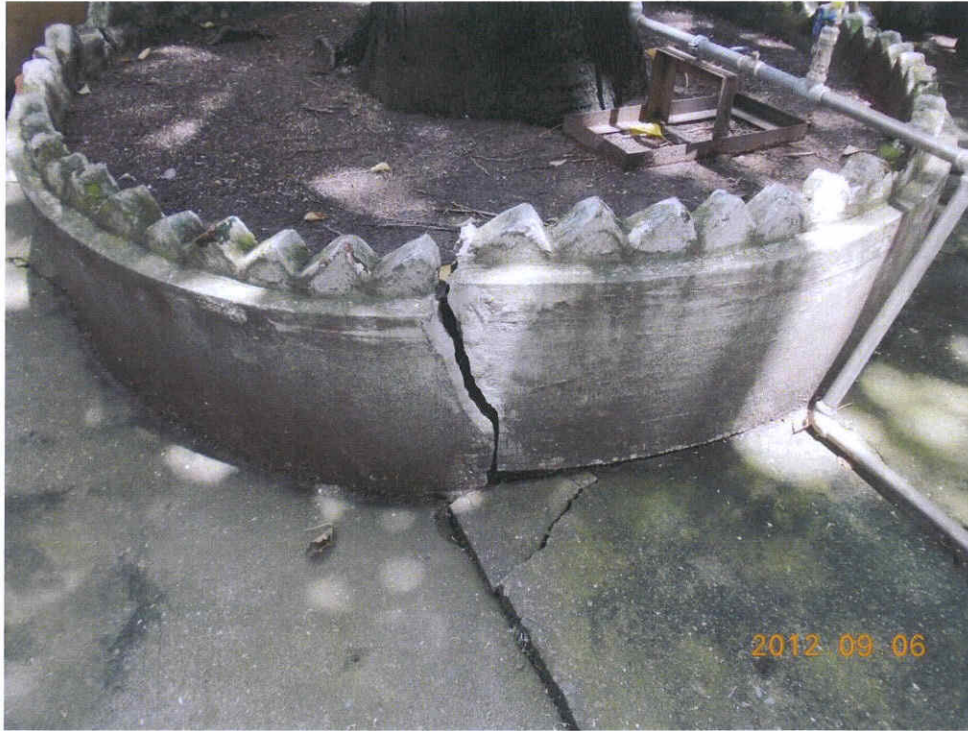
Fig. 4 Cracks are getting worse during inspection on 6 th September 2012.
