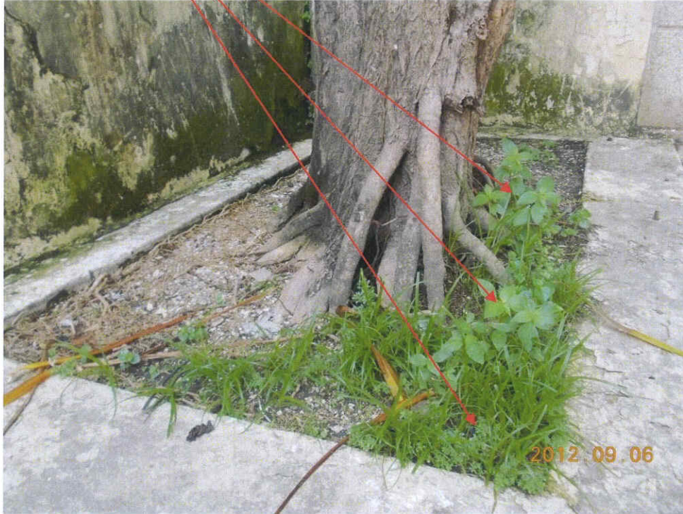
Fig. 2 Some weeds appear at the planter, recommend to clear all these weeds away from the planter.
