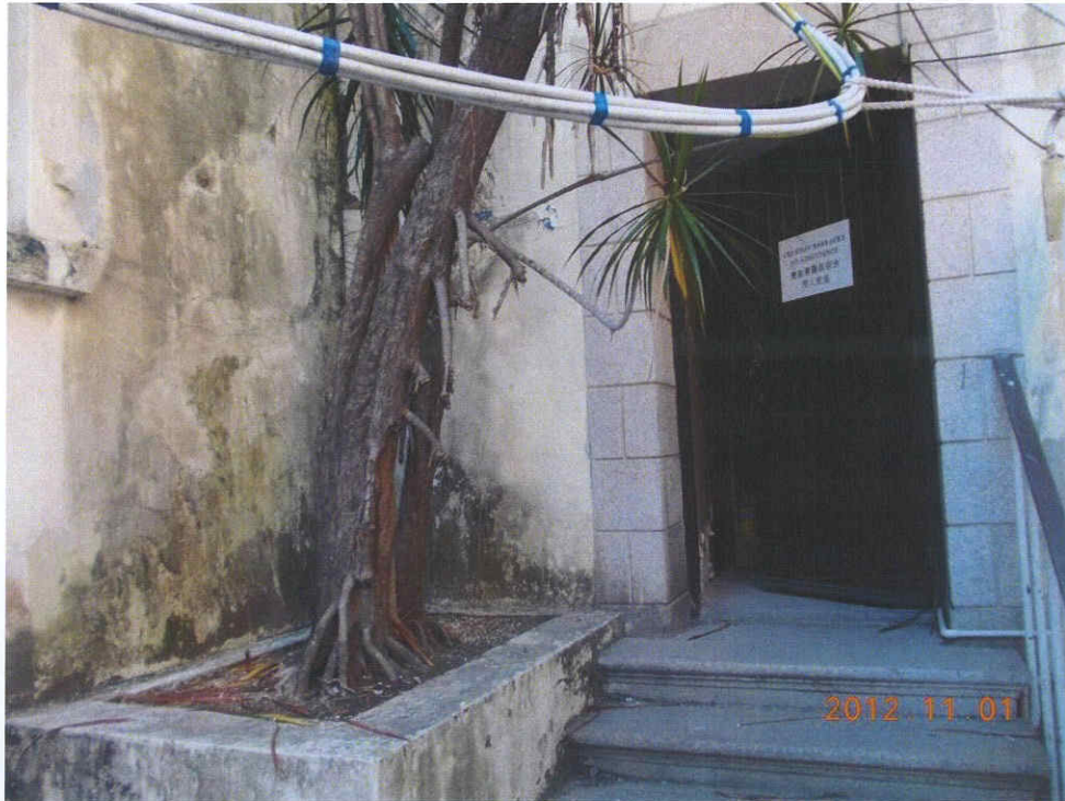
Fig. 4 The wooden door keeps opened at the time of inspection.
