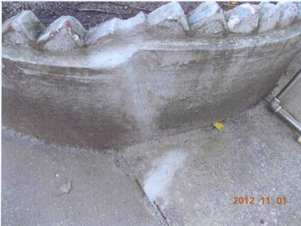
Fig 3 The cracks in question are well-repaired. No more new cracks have been found at the time of inspection.
