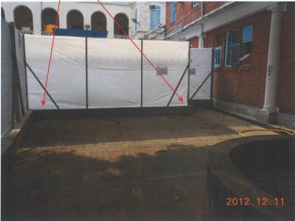
Fig. 3 A root-wall is newly built inside the cordon zone. Cleanliness of the site is acceptable.
