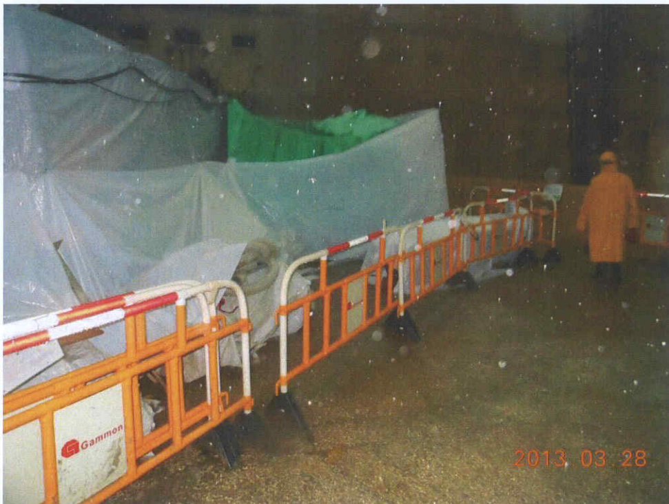
Fig. 5 It is raining at the time of inspection, the site outside the cordon zone is clean and tidy.
