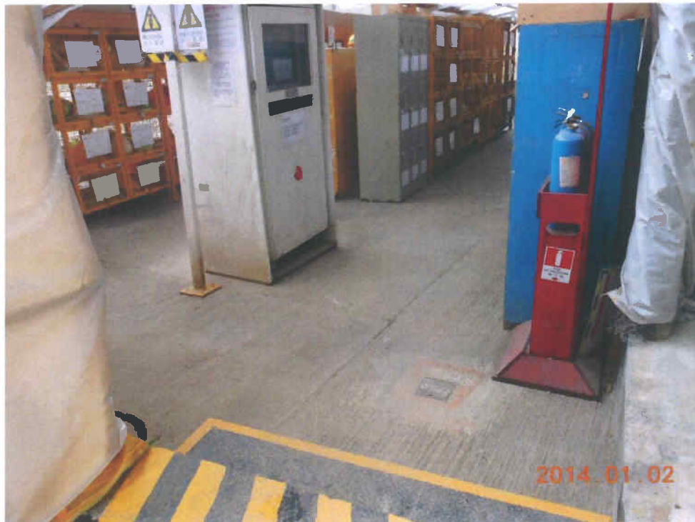
Fig. 9 The store-room near Tree-5 is clean and tidy.
