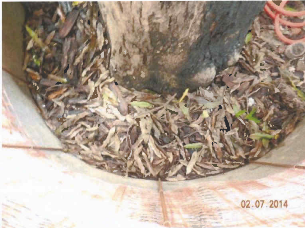
Fig 2. The root collar of Tree-5 is good. The planter is full of mulch.
