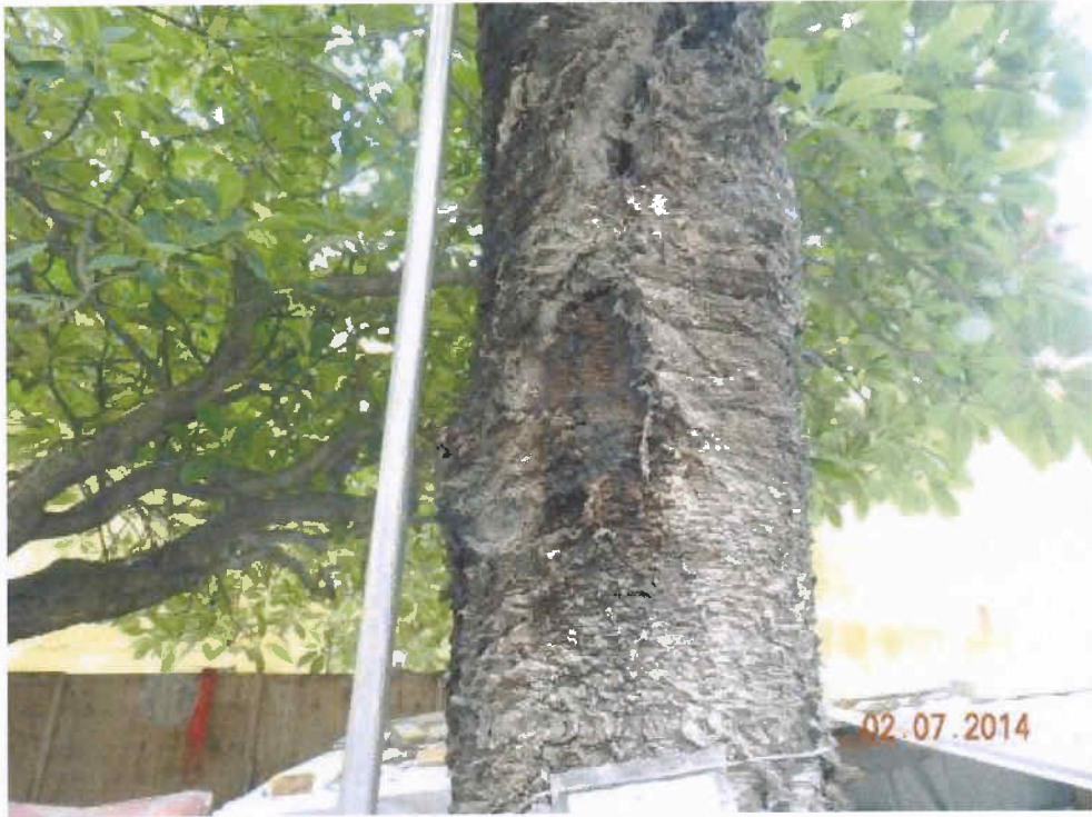
Fig. 4 No signs of sap flow have been detected again on the cavity.
