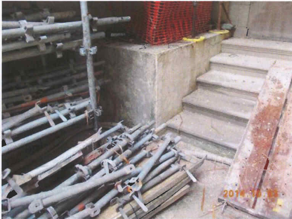
Fig. 8 Many metal tubes are placed near the planter.
