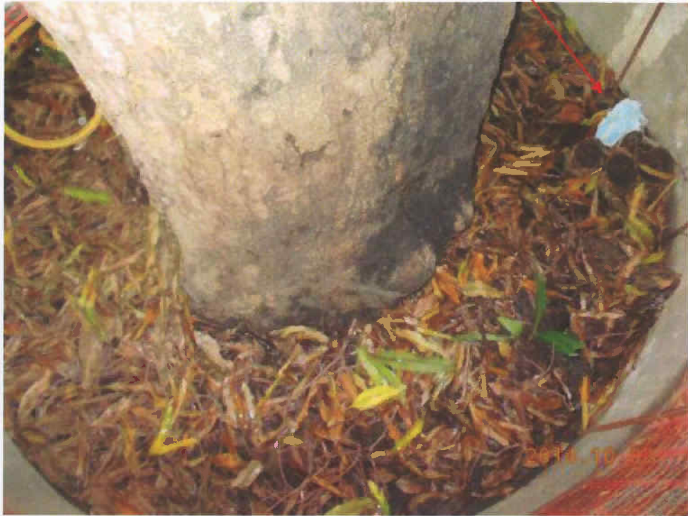
Fig 2. The root collar of Tree-5 is normal. A few litter has been found at the planter.
