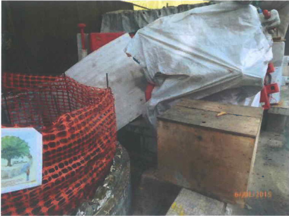
Fig. 8 Many bulky items are placed near the tree.
