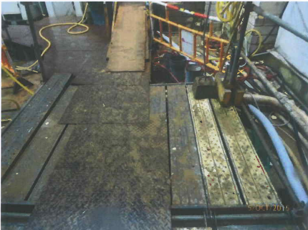
Fig. 11 Cleanliness of the site outside the cordon zone is acceptable.
