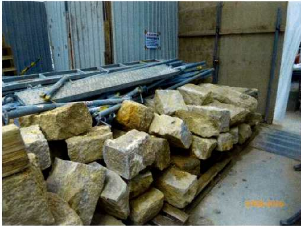
Fig. 10 Many bulky construction items are placed near the cordon zone.
