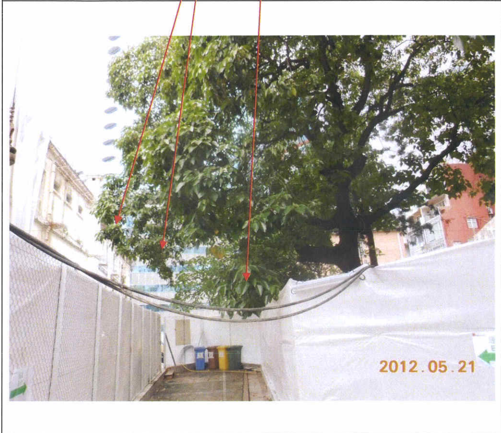
Fig. 6 Some lower branches and leaves are too close to the fence of the cordon zone, we recommend to trim these branches and leaves.
