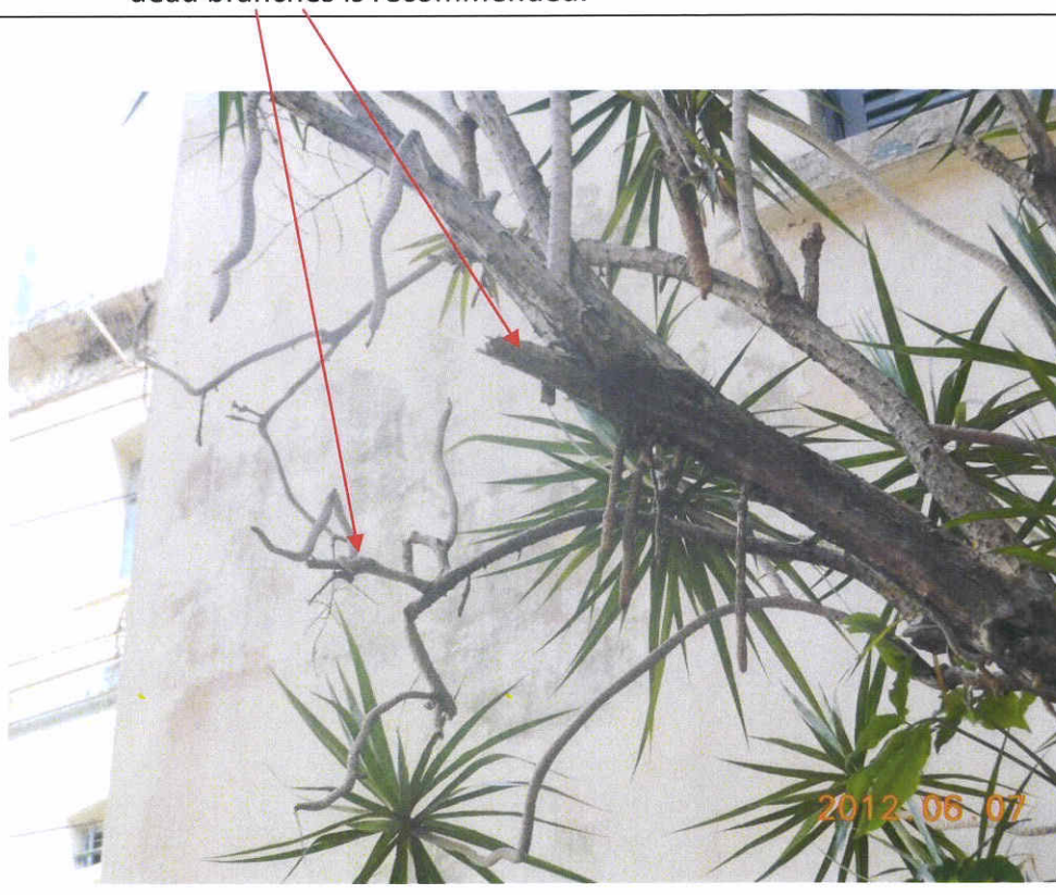
Fig. 5 Some dead branches appear on the tree. Trimming of these dead branches is recommended.
