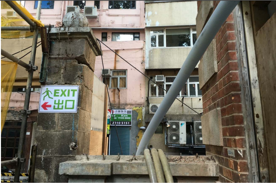
Above, photograph taken on 25 th January 2016, showing the fence was missing.
