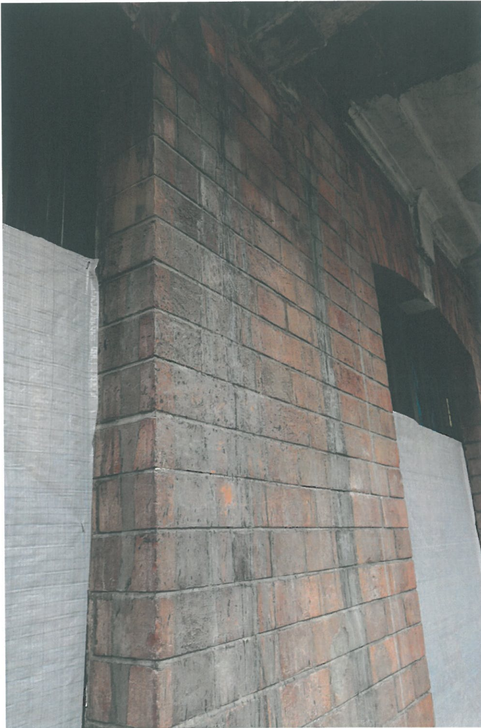
Above, photo taken on 18 th March 2016, showing spilt concrete on the Block 9 Magistracy Terrace (2/F West elevation).
