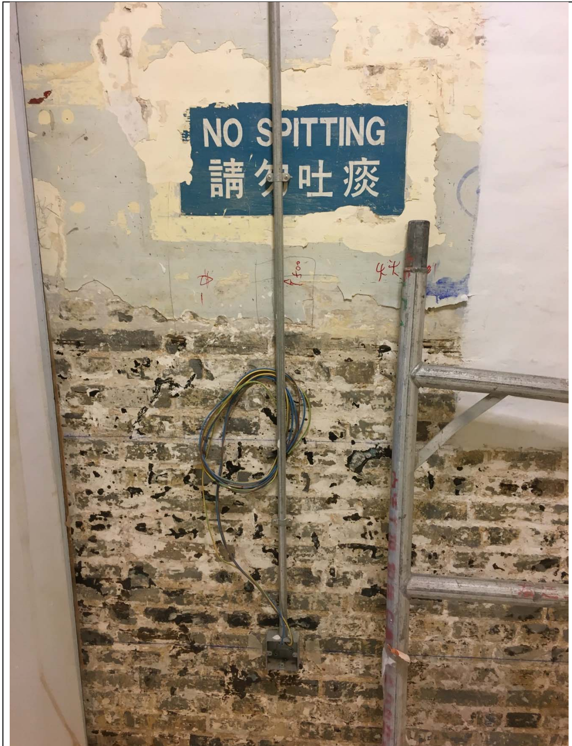
Above, photograph taken on 2 nd February 2016, protection to the painted sign “NO SPITTING 請勿吐痰” was removed and a conduit was directly fixed on the painted sign.
