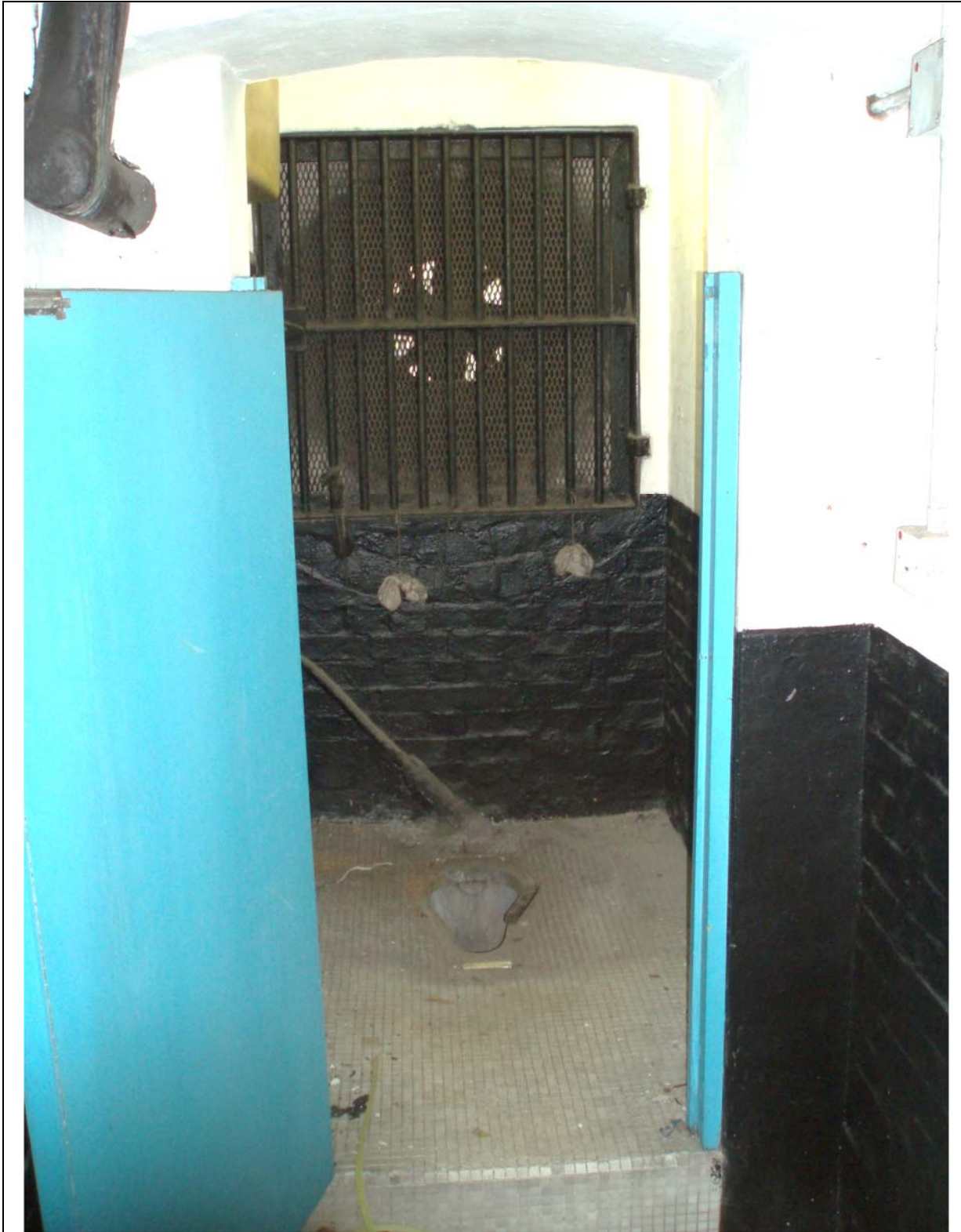
Above, photograph taken on 27 th July 2009, showing the overall view of the holding cell toilet.
