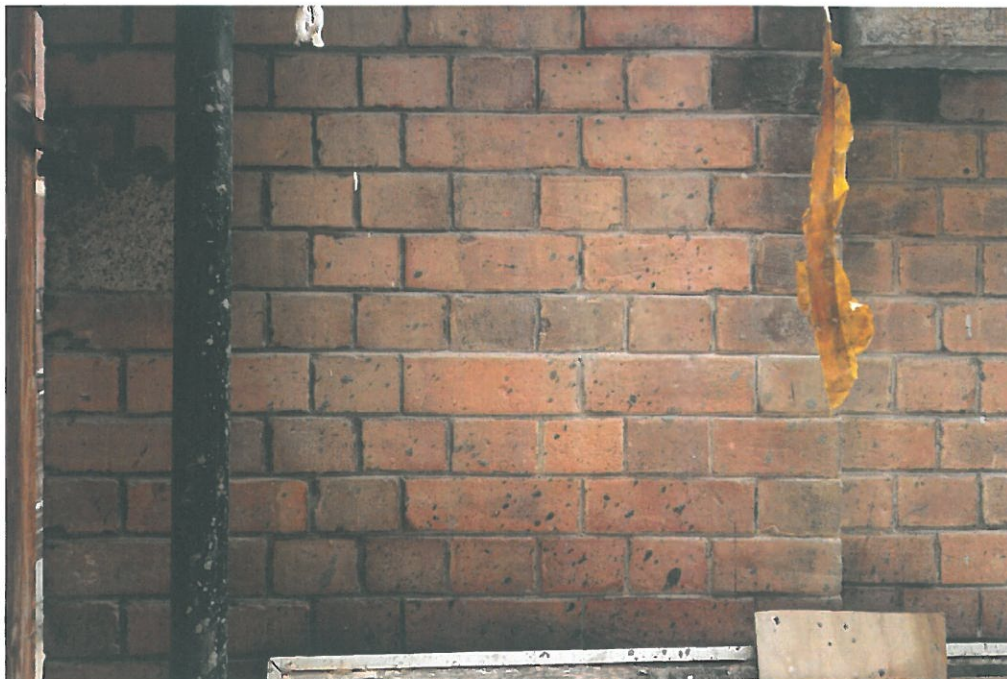
Above, photo taken on 18 th March 2016, showing the close-up of the spilt concrete on the boundary wall opposite Block 9 Magistracy West elevation.
