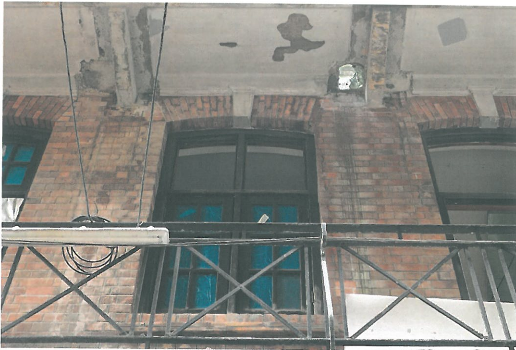
Above, photo taken on 18 th March 2016, showing spilt concrete on the Block 9 Magistracy West elevation (1/F).
