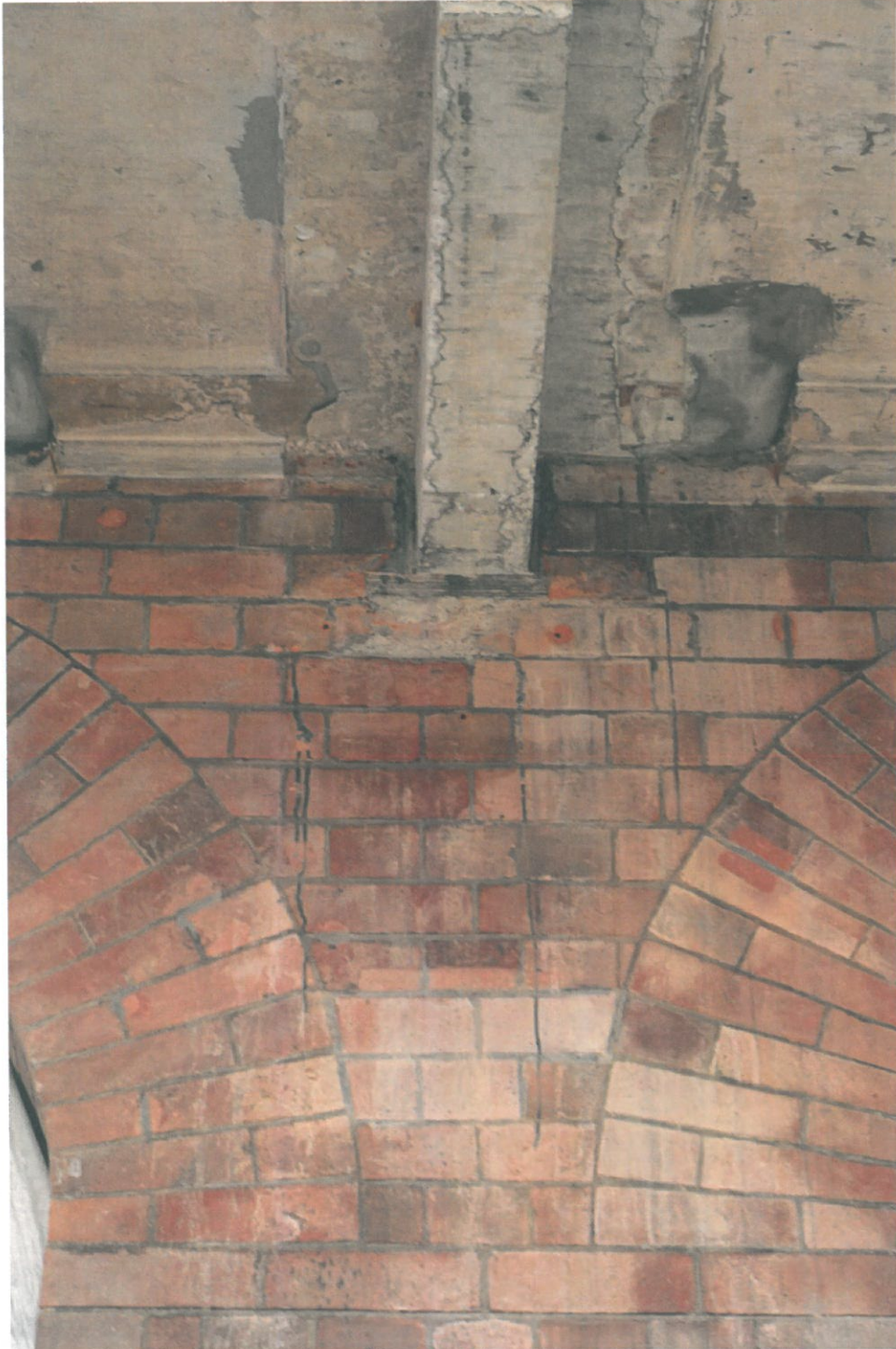
Above, photo taken on 18 th March 2016, showing spilt concrete on the Block 9 Magistracy West elevation (G/F).
