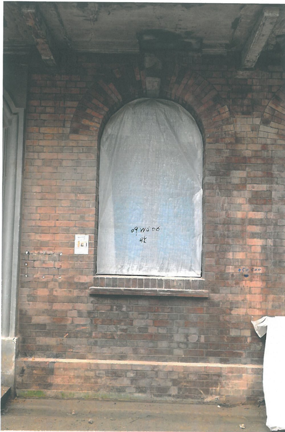
Above, photo taken on 18 th March 2016, showing spilt concrete on the Block 9 Magistracy West elevation (G/F).
