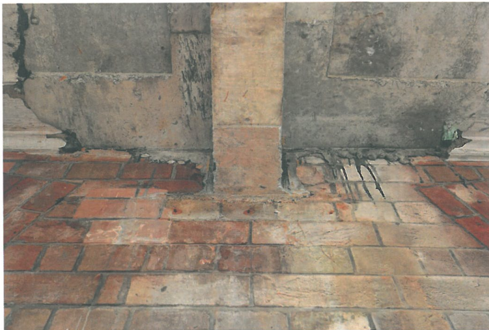
Above, photo taken on 18 th March 2016, showing spilt concrete on the Block 9 Magistracy Terrace (2/F West elevation).
