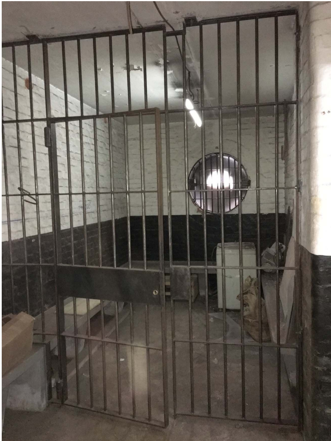
Above, photograph taken on 25 th February 2016, the conduits, lighting, mesh and fan on the window, paint on the metal gate were incorrectly removed. Removal of mesh had damaged adjacent brickwork.
