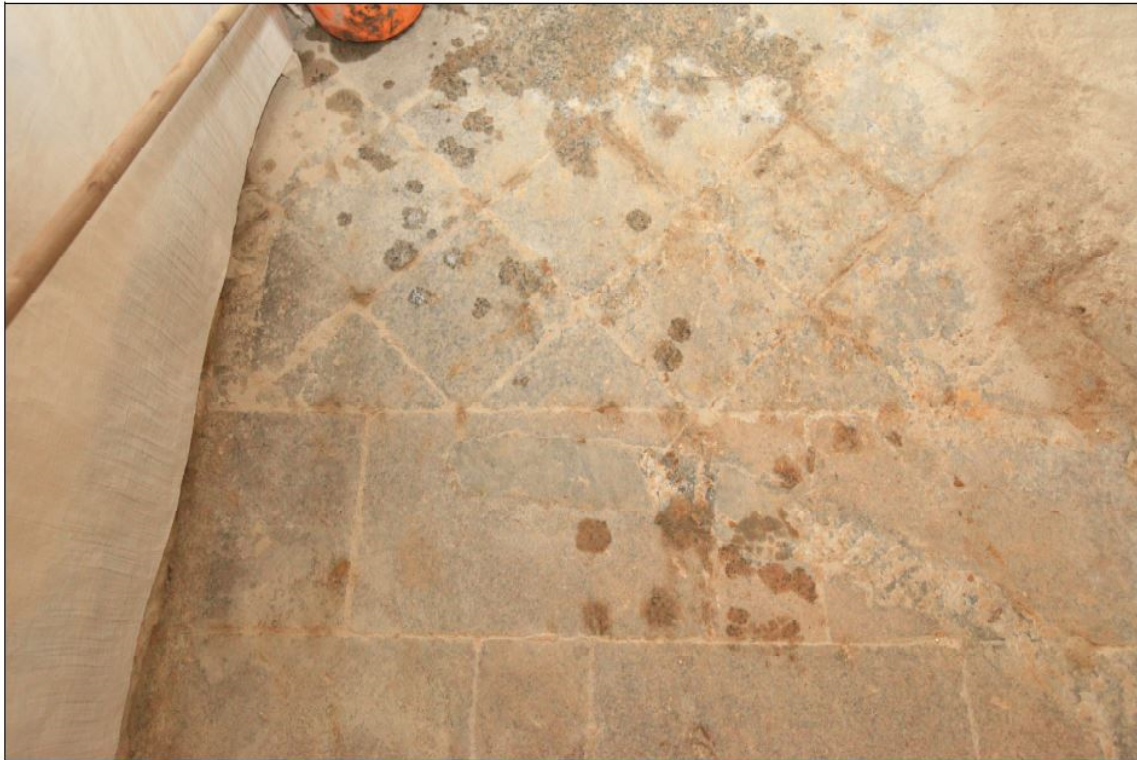
Photograph taken on 22 nd August 2013 by the Management Contractor, showing the granite border at the west archway.
