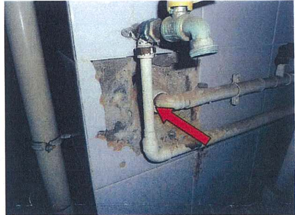
Photo 2. Embedded hot water pipe was insulated with uPVC material
