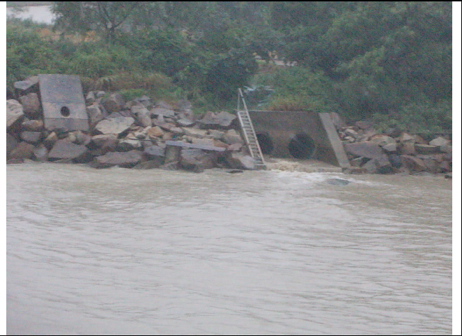
Photo 2. Muddy water was observed near W1.
