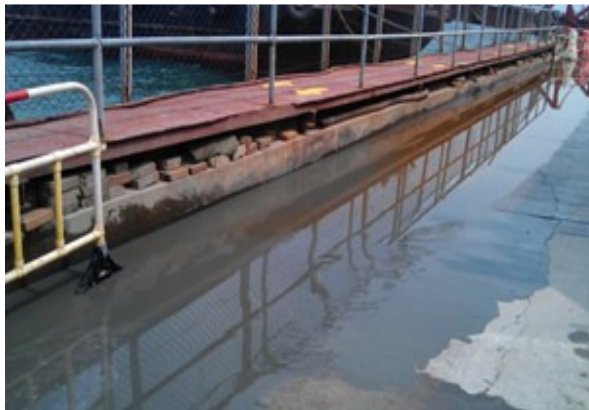
Photo 1 Water with sand was accumulated along the path near the entrance.
