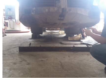
Photo 2 The oil leakage was found from equipment during the maintenances process.
