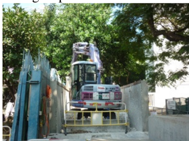
Photo 1 No cement mixing process was found during inspection.
