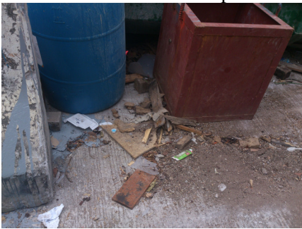
Photo 1 The general waste was found accumulated in the workshop area.
