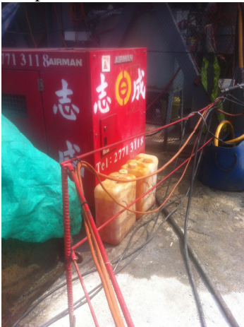
Photo 1 Chemical containers were found to be without drip trays near the compressor area.
