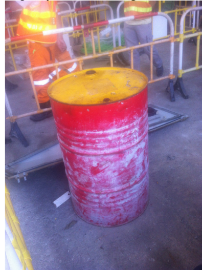
Photo 2 Chemical container was found without a drip tray in the welding area.
