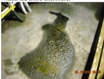
Photo 1 Oil spot was observed on the ground within the noise enclosure.
