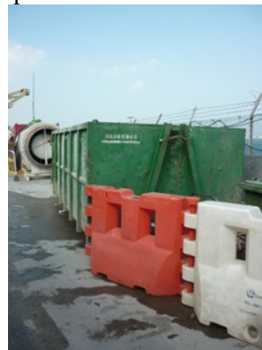
Photo 2 A damage skip was found next to the stockpiles
