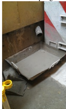
Photo 2 Wastewater from concrete sampling was stored in an unsuitable container. The waste water may overflow during the concrete sampling.
