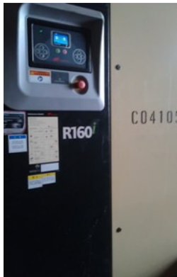
Photo 1 No noise label was provided for an air compressor inside the noise enclosure.
