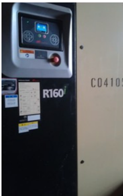
Photo 1 No noise label was provided for an air compressor inside the noise enclosure.
