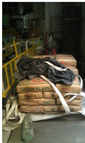
Photo 4 Concrete bags were found without cover
