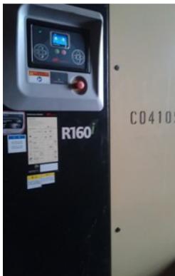
Photo 1 No noise label was provided for an air compressor inside the noise enclosure.
