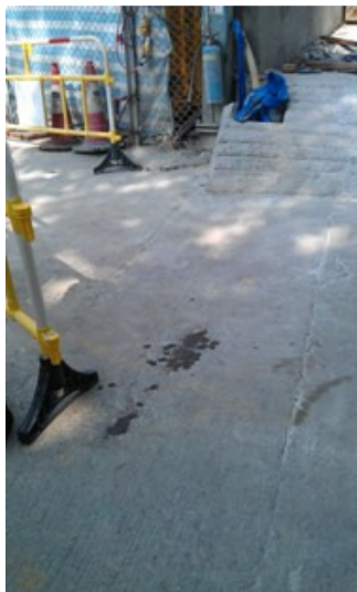
Photo 1 Oil stains were found in the access near the mobile crane
