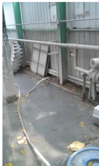
Photo 4 The concrete wastewater was accumulated near the RE's car park
