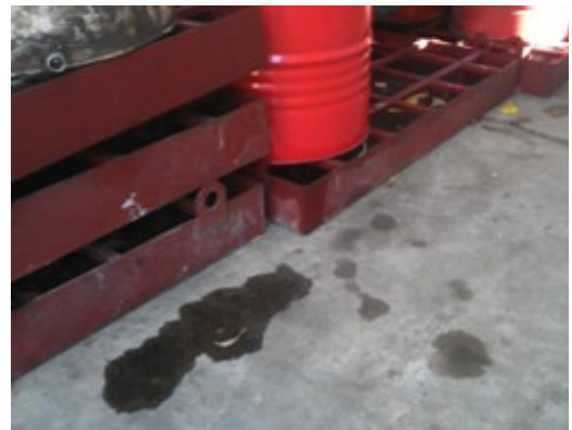
Photo 2 Oil stains were found near drip trays
