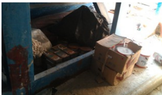
Photo 1 Some chemical drums were found without drip trays under the Aqua. Sedimentation tank
