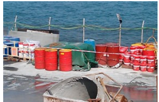
Photo 2 No dript trays were provided for some chemical drums near stockpiles.
