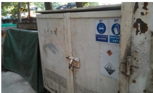
Photo 1 The storage area for rechargeable battery was not locked.
