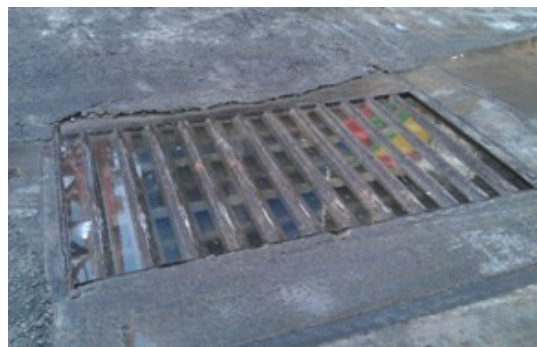
Photo 4 Water ponding was found in the abandoned washing vehicle facilities
