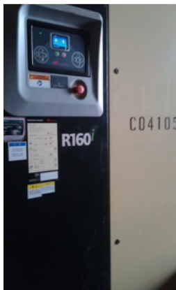
Photo 1 No noise label was provided for an air ompressor inside the noise enclosure.
