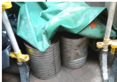
Photo 2 Some chemical drums were found without drip trays and chemical labels in access between noise enclosure and DSD treatment plant.
