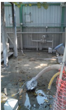
Photo 3 The concrete wastewater was accumulated near the RE's car park.
