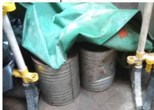
Photo 2 Some chemical drums were found without drip trays and chemical labels in the access between noise enclosure and DSD treatment plant.
