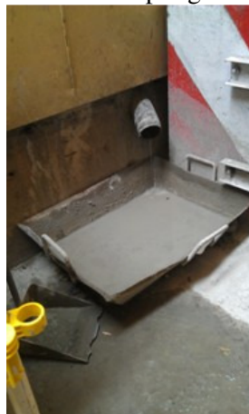
Photo 2 Wastewater from concrete sampling was stored in an unsuitable container. The waste water may overflow during the concrete sampling.
