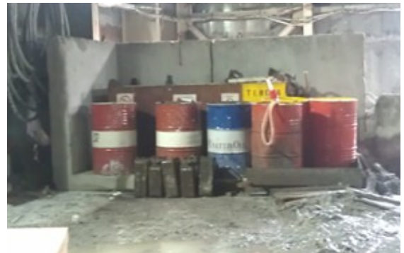
Photo 2 Chemical drums were found without chemical labels and drip trays in the noise enclosure.
