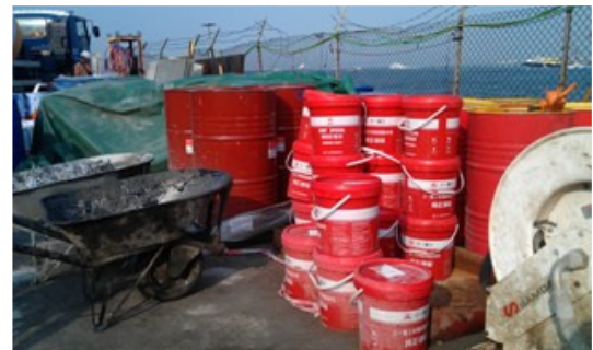
Photo 2 No dript trays were provided for some chemical drums near stockpiles.
