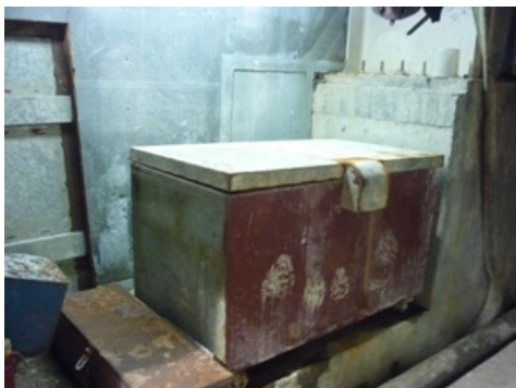
Photo 5 Water accumulated and trashes were found in the skip in the noise enclosure
