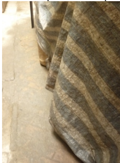
Photo 2 Another chemical drum was found on access near the DSD plant without drip tray
