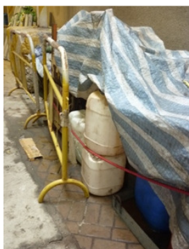
Photo 1 Chemicals without drip tray were found on the access near the noise enclosure
