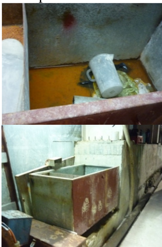
Photo 1 Water accumulation and trashes were found in skip inside the noise enclosure
