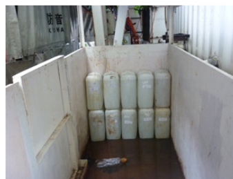
Photo 2 Water accumulation was found in drip tray since last inspection
