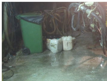
Photo 4 Chemicals without drip tray were found in the tunnel adit.
