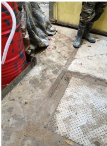
Photo 4 Oil droplets were found near the noise enclosure
