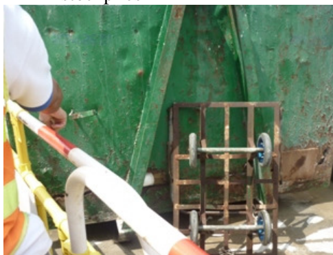
Photo 4 A broken skip was found near stockpiles
