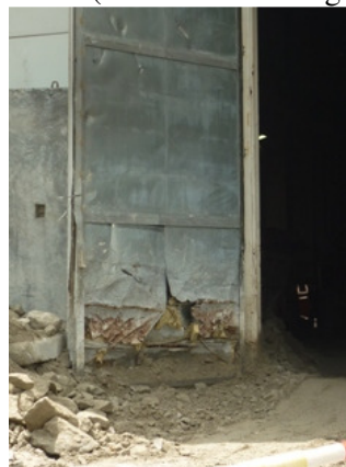
Photo 2 The door of noise enclosure was found broken.(Taken on 14 th August 2012)
