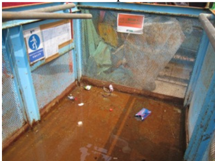
Photo 9 Stagnant pool and leaves were found around the workshop
