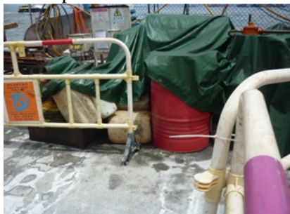
Photo 1 Some chemical containers were found without labels and drip tray near stockpiles
