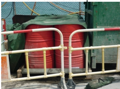
Photo 1 Drip tray was provided to the chemical containers near the stockpiles
