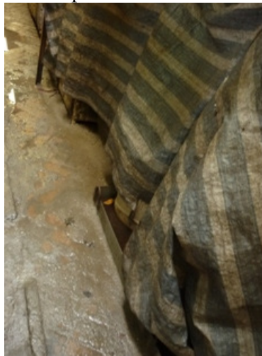
Photo 2 Oil droplets were found next to drip tray near the DSD plant
