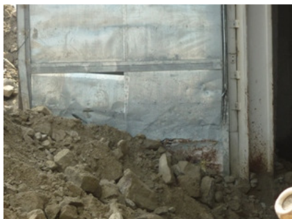
Photo 1 The door of noise enclosure was found broken.
