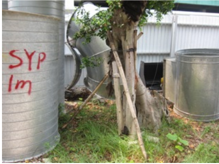
Photo 7 The transplanted tree T003 was found without protective fence since last inspection
