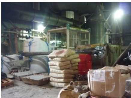
Photo 3 Cement bags without properly cover
