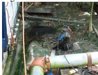
Photo 4 Water accumulation was found behind the storage container
