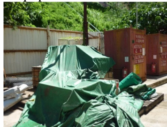
Stagnant water pools were found on the shelter of equipments in the workshop area.
