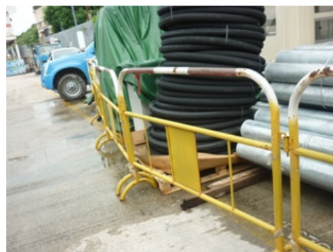
Photo 2 Water leaking and accumulated were found around the adjacent contractor's site office
