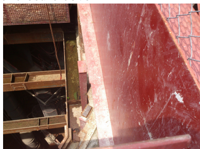
Photo 1 Stagnant water was found in skip on noise enclosure cover
