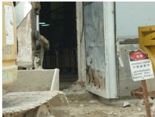
Photo 2 The door of noise enclosure was found broken.
