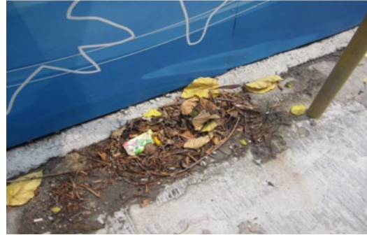
Photo 8 Stagnant pool and leaves were found around the workshop
