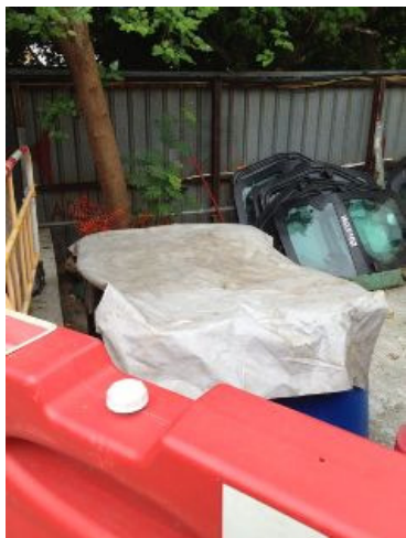
Photo 3 Tarpaulin had been provided to barrels near the DG Storage to prevent water accumulation
