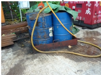
Photo 7 Oil stains in workshop area was cleared
