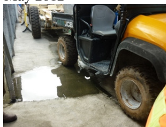
Photo 7 Water accumulation was found near the plant in front of site office. The dilapidation roof of site office was found to avoid the water leakage in PTW since inspection on 29 May 2012
