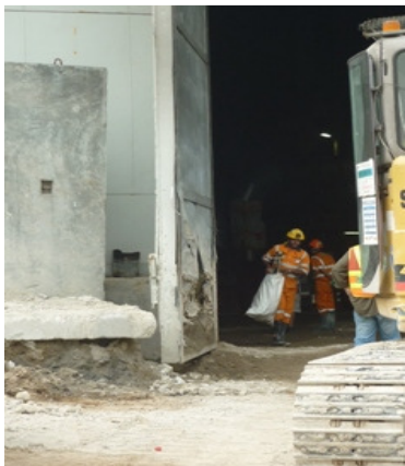
Photo 1 The door of noise enclosure was found broken.
