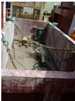
Photo 1 Stagnant water was found in skip on noise enclosure cover
