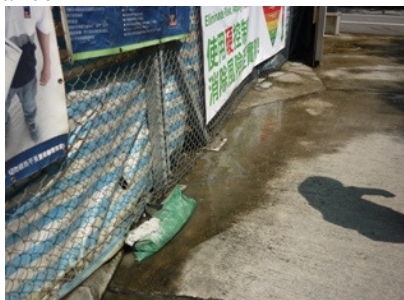
Photo 1 Water ponding was found near the site entrance
