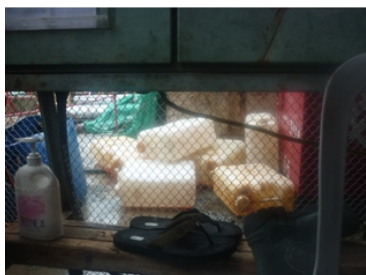
Photo 1 Some chemical drums were found without suitable labels and drip tray next to air compressor near the mobile crane.
