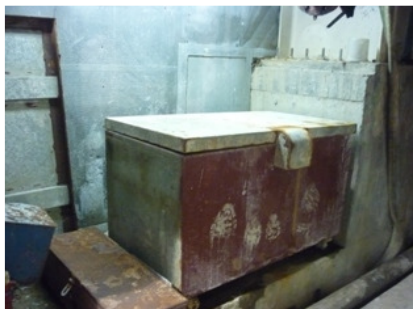
Photo 5 Water accumulated and trashes in the skip in the noise enclosure
