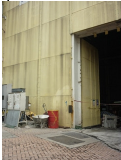
Photo 1 Chemical barrel was found without drip tray near the door of noise enclosure
