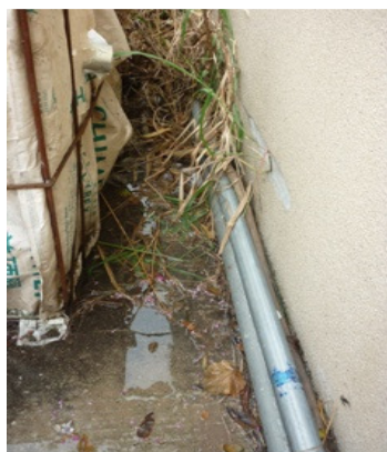
Photo 1 Water leaking and accumulated were found around the adjacent contractor's site office
