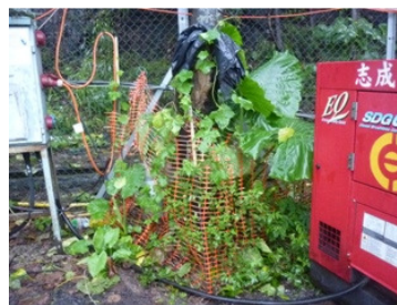
Photo 2 Some chemical drums were found near the retained tree near plants stockpiles in workshop.
