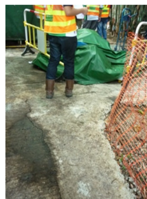
Photo 9 Oil remaining was found near the chemical storage
