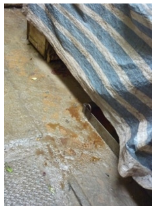
Photo 4 Oil droplets was found near the noise enclosure
