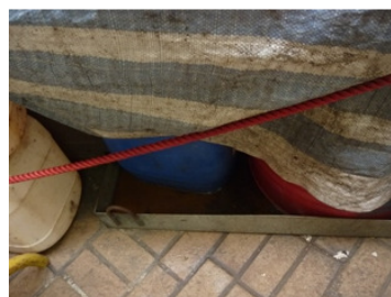
Photo 2 Some soil droplets were found near stockpiles in the noise enclosure.
