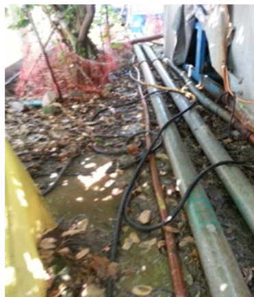
Photo 2 Water accumulation was found behind the sedimentation tank
