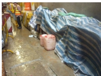
Photo 1 Chemicals without drip tray were found on the access near the noise enclosure
