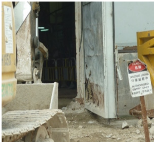
Photo 2 The door of noise enclosure was found broken.
