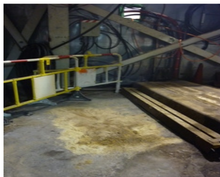
Photo 2 The waste oil was cleared with oil absorbents.
