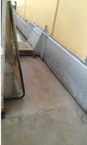
Photo 3 Water accumulation was found on path next to noise enclosure.
