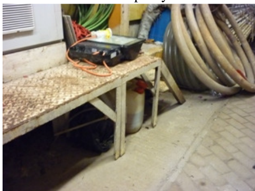
Photo 1 A chemical drum was found without chemical label and drip tray
