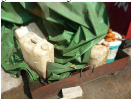
Photo 7 Waste oil was accumulated in drip tray of generator at storage area
