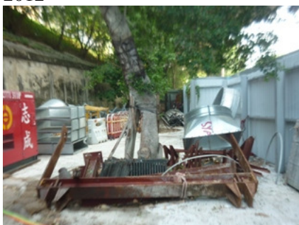
Photo 1 Construction materials were stored too close to the tree (T003 (T)) in Storage area since inspection on 24 October 2012
