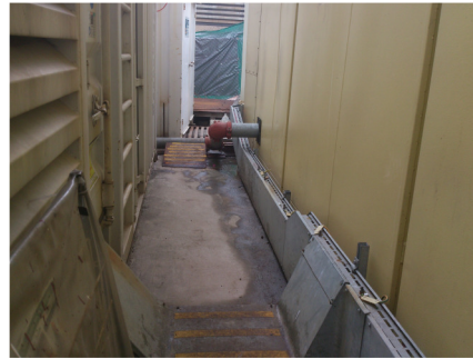
Photo 2 Water accumulation was found on path next to noise enclosure.
