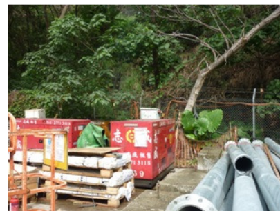
Photo 6 Some white smoke was observed from generator in storage zone.
