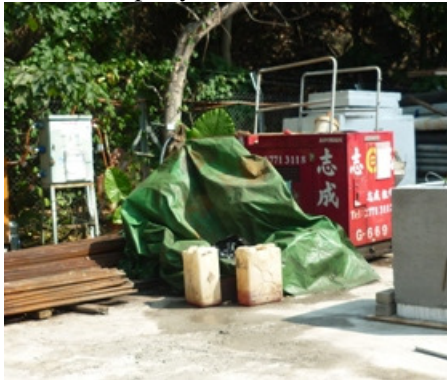
Photo 3 Some known chemical containers were found next to the generator without drip tray and labels.
