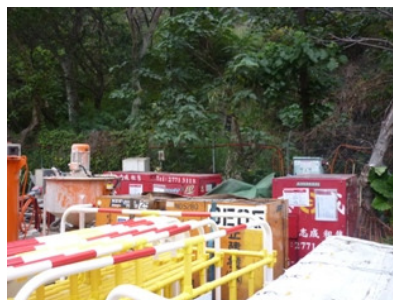
Photo_F 2 No white smoke was exhausted from the generator.
