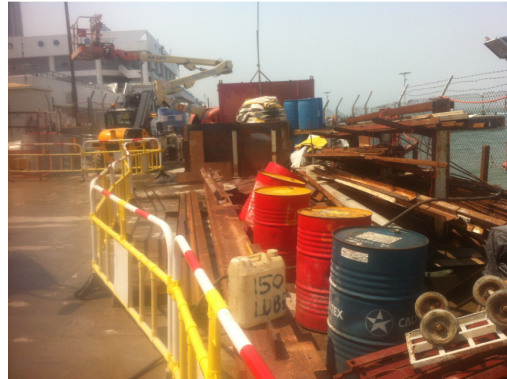
Photo 2 Chemical barrels were found to be without drip trays outside the noise enclosure area
