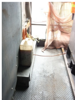
Photo 1 A chemical container was found near the generator at the first platform without label.
