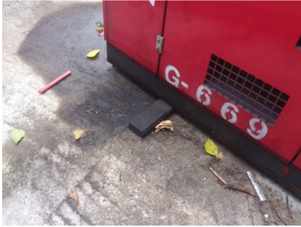
Photo 4 The oil stains were found on the ground near the generator.
