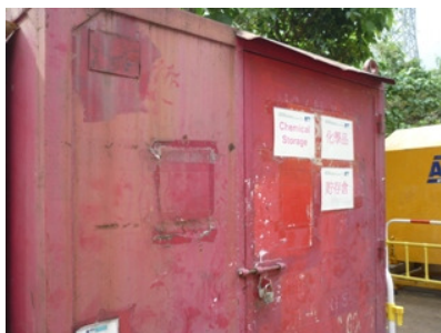
Photo 3 The chemical storage was found without chemical storage list since the site inspection undertaken on 30 th October 2012
