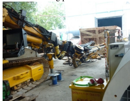
Photo_F 2 The chemical with green colour under the drilling plant was cleared
