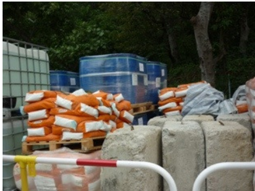
Photo 5 Dusty materials were not covered properly.
