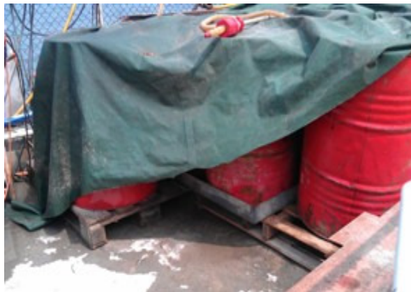
Photo 2 Chemical barrels were found to be without drip trays outside the noise enclosure area.
