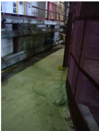
Photo 3 Water accumulation next to air compressor in noise enclosure was cleared.
