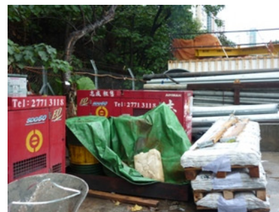
Photo 8 Some white smoke was observe from generator in storage zone
