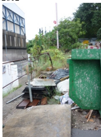
Photo 4 Some trashes were found near the rubbish skip in storage area since the site inspection undertaken on 13 th November 2012
