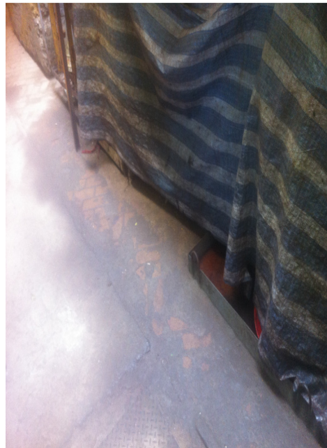
Photo 2 Waste oil was found near the noise enclosure of the inner entrance
