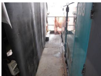
Photo_F 1 The chemical container near the generator at the first platform was removed.
