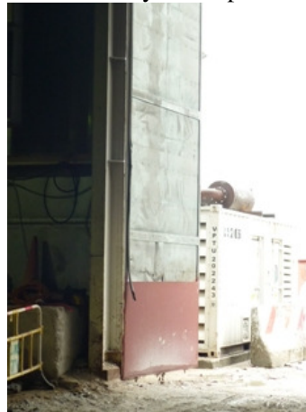
Photo 6 The door of the noise enclosure had been cover by metal plate
