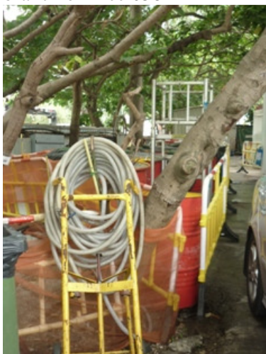
Photo 5 Non-use water plastic pipe hang from the branch of Tree 038
