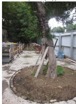
Photo_F 2 The construction materials were moved away from the tree (T005 (T)) and tree (T84(R)) in storage area.
