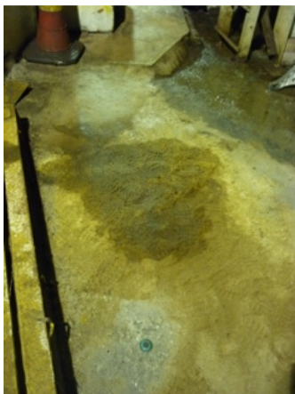
Photo 3 Some sand mix with oil was found inside noise enclosure
