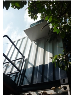
Photo 2 An water dripping air conditioner was found next to new chemical storage.
