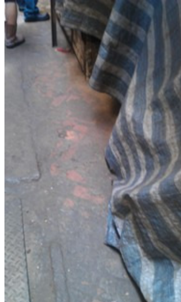
Photo 4 Waste oil near the noise enclosure of the inner entrance was cleared
