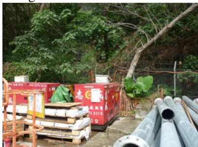
Photo 5 Some white smoke was observed from generator in storage zone.
