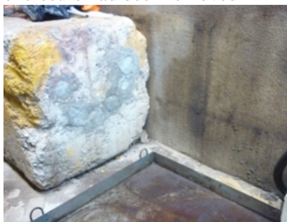
Photo 2 The unknown chemical near the noise enclosure had been removed
