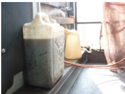
Photos 3 A chemical container was found near the generator at 1 st platform without label
