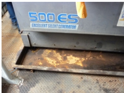
Photo_F 1 Waste oil accumulated in drip tray of generator at the first platform was cleared.
