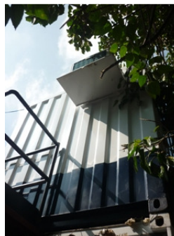
Photo 2 An water dripping air conditioner was found next to new chemical storage.
