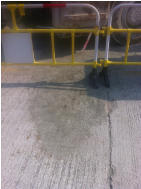
Photo 1 Loose sediment was found on the pavement surface area near the site offices
