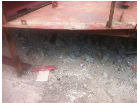
Photo 2 Rubbish and cigarettes butts were found inside the site area.
