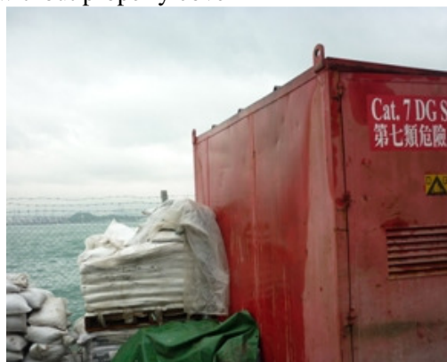
Photo 4 Some dusty material were found without properly cover
