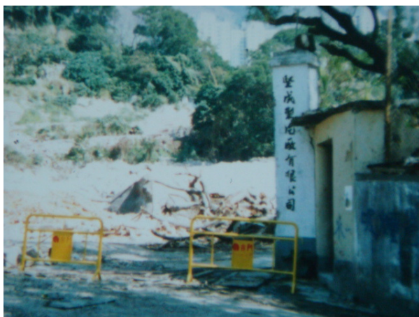
Photo a6 Demolition and dismantling of Jiancheng Film Studio in the 1980s
