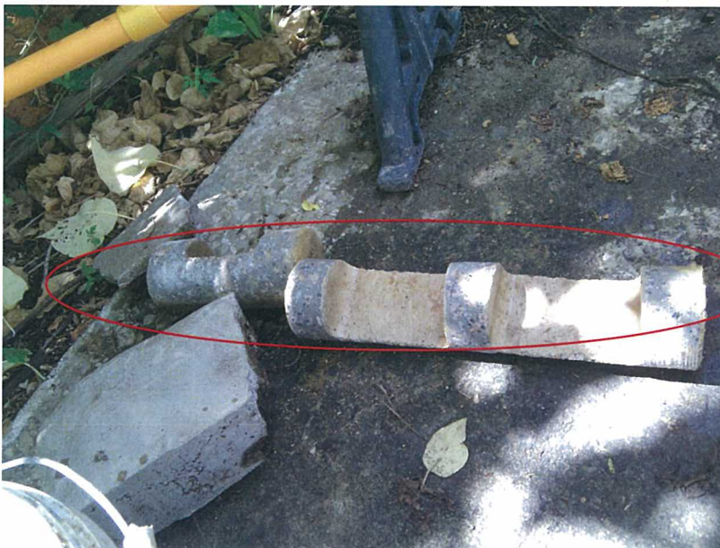
Extracted core samples, mark W1-1 and W1-2, revealed the wing wall of pillbox was constructed by two rows of concrete hollow blocks
