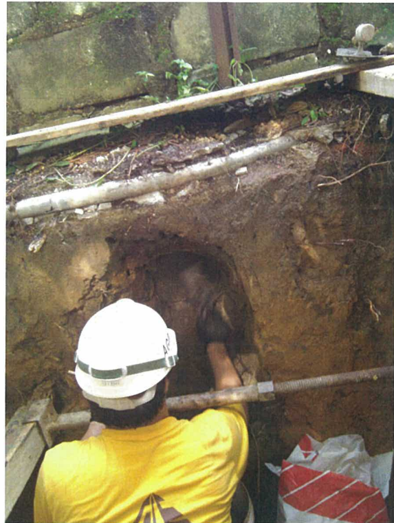
Core-hole and bolt hole were reinstated by FORSOC Renderoc HB40 immediately after inspection
