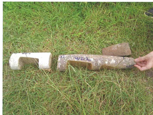
Extracted core samples, mark W2-1 and W2-2, revealed the wall of pillbox was constructed by two rows of concrete hollow blocks
