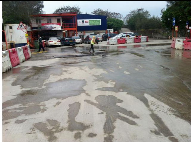
Photo 3. The floor area was watered by site workers at the exit point.
