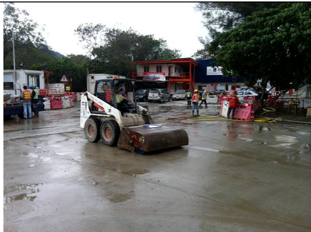
Photo 5. A Bob Cat with sweeper was used to clean out the mud deposited on the paved road instead of water truck.
