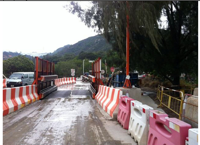
Photo 4. The Contractor had provided a workable and effective wheel washing system at the exit point of the site, comprising high pressure water jets.
