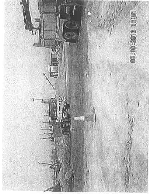
Photo 161006_001 (Dry mud zone) (Improved)
