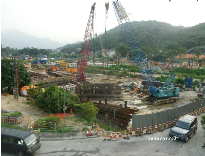
Photo 3: Overview of the construction works site which significant dust emission was not observed (Date: 23 July 2014)
