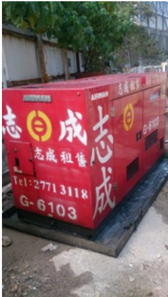
Photo 1 Stagnant water was found inside a drip tray for a red generator.
