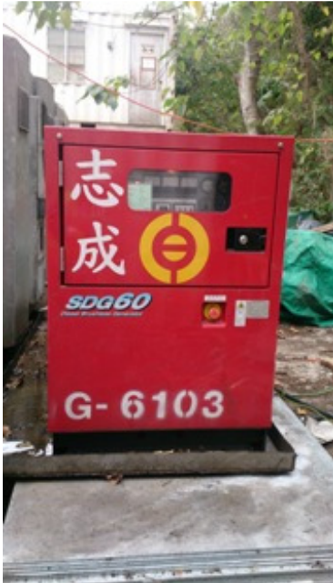
Photo 1 Stagnant water was found inside a drip tray for a red generator
