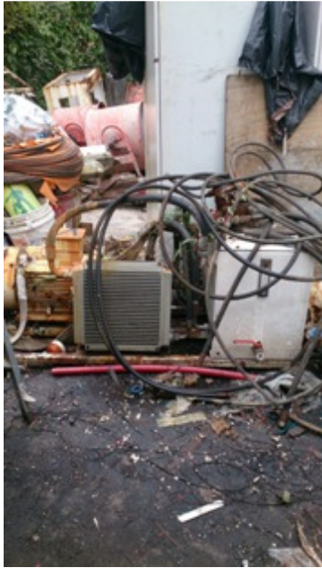
Photo 2 An oil stain was found near electricity boxes
