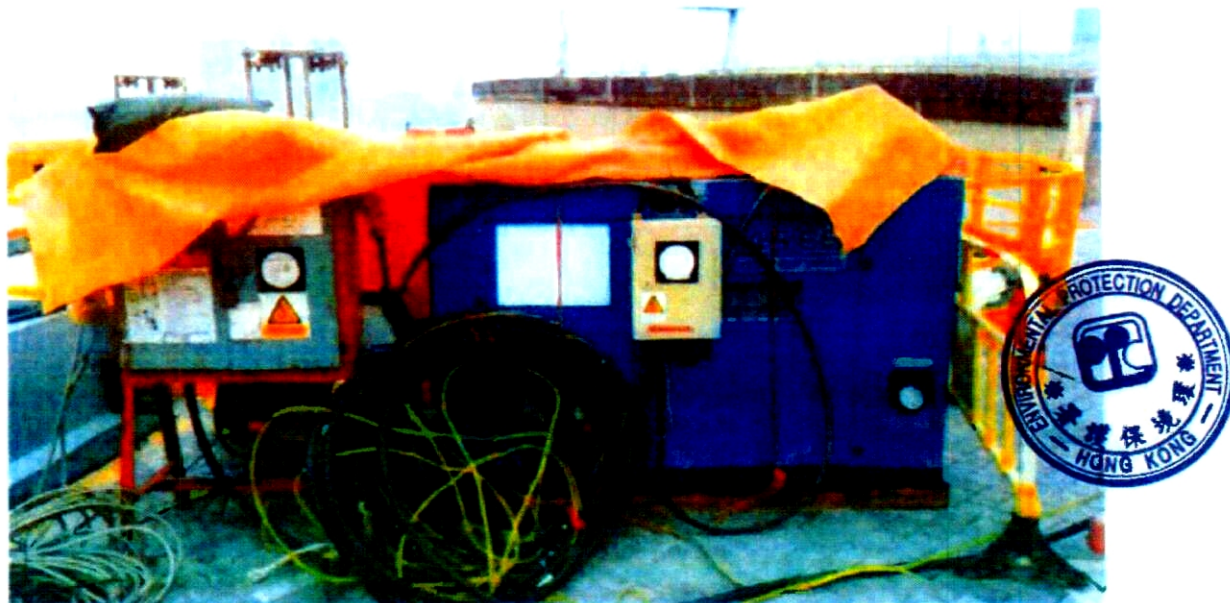
發電機，備有優質機動設備標籤顯示聲功率級 \leq 89 分貝(A) Generator, with Quality Powered Mechanical Equipment Label showing a sound power level of \leq 89 dB(A)
