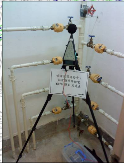
Measurement Location in GN5 (Tower 5, Park Avenue): Water Meter Room, 2 nd Floor
