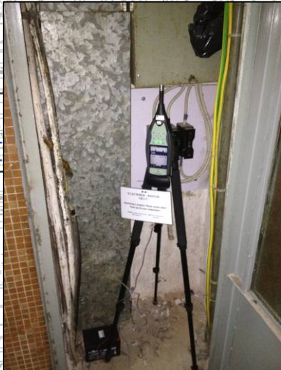
Alternative Measurement Location for GN7 (Tai Shing Building (Block H Cosmopolitan Estates): Electricity Meter Room in 1 st Floor
