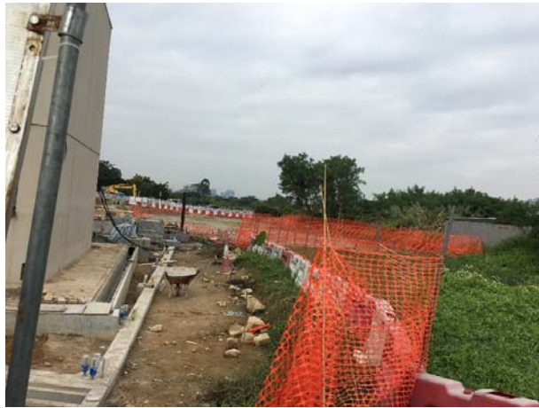
Plate 7 Access path blocked by project-related works at Point Count Location SSS-3/P6
