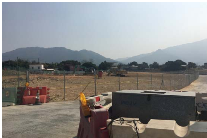
Plate 8 Project-related construction works for SSS/ERS were observed near Point Count Location SSS-1/P1
