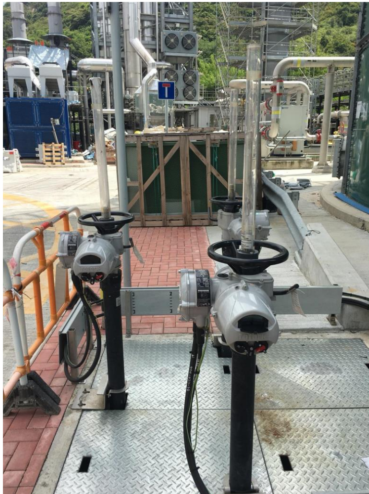
Penstocks are in close position under normal operation.
