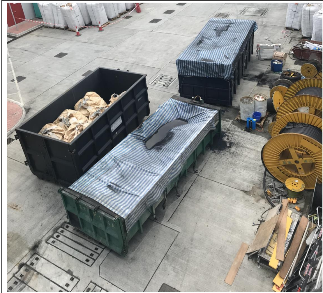
The Activate Carbon (ACs) were standby for replacement on site in mid-September 2018.
