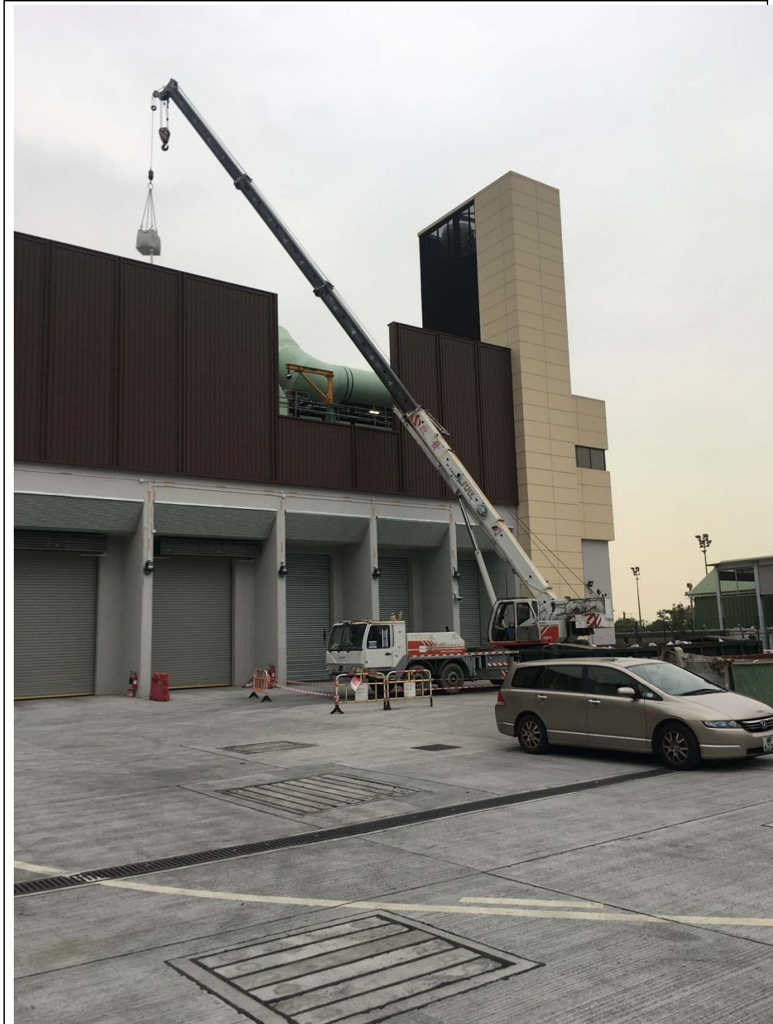
The AC bags were being lifted to roof of the Building 2 and ready for replacement.
