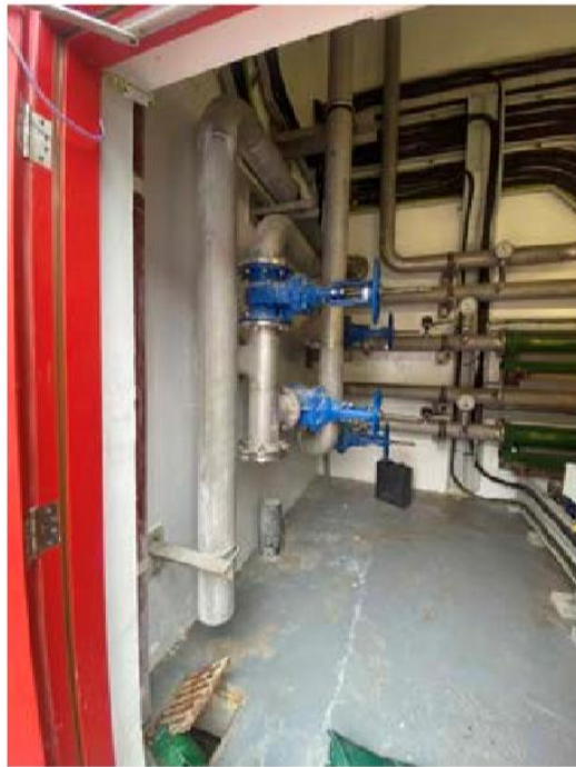
Figure.3 Misalignment of overflow pipeline to the drain pit inside the TE pump room
