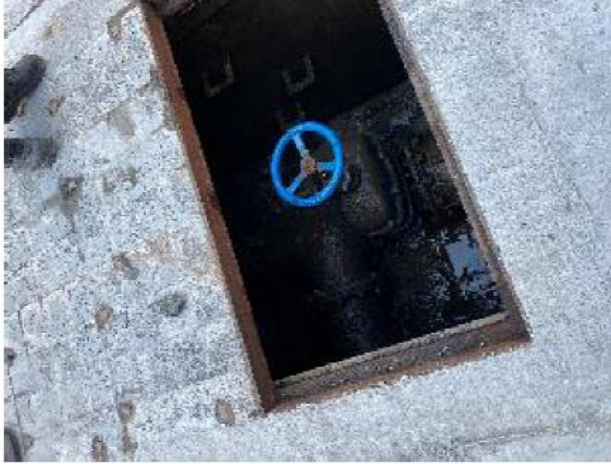
Figure.5 Preventive action: AD tank from stormwater 3-way gate valve is closed
